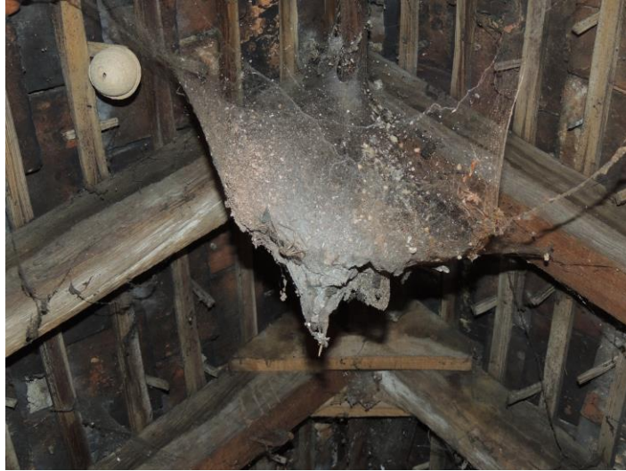
Photo 13: Note cobwebs in second loft
