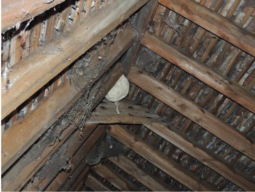
Photo 16: Note cobwebs along ridge of third loft
