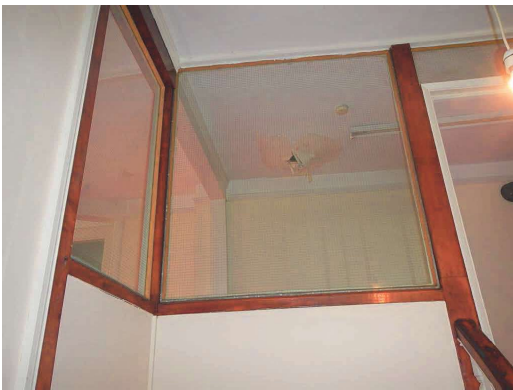
25. School-era partitioning around stairs
