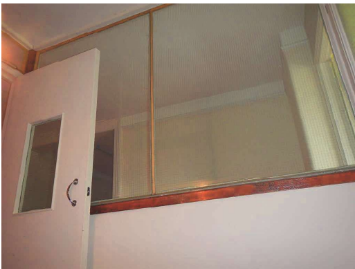
26. School-era partitioning around stairs
