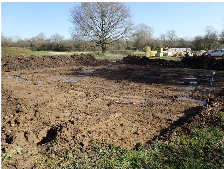
Plate 6: Trench 9, view to north-east, scale 1m. Ground reduction did not attain the underlying geology
