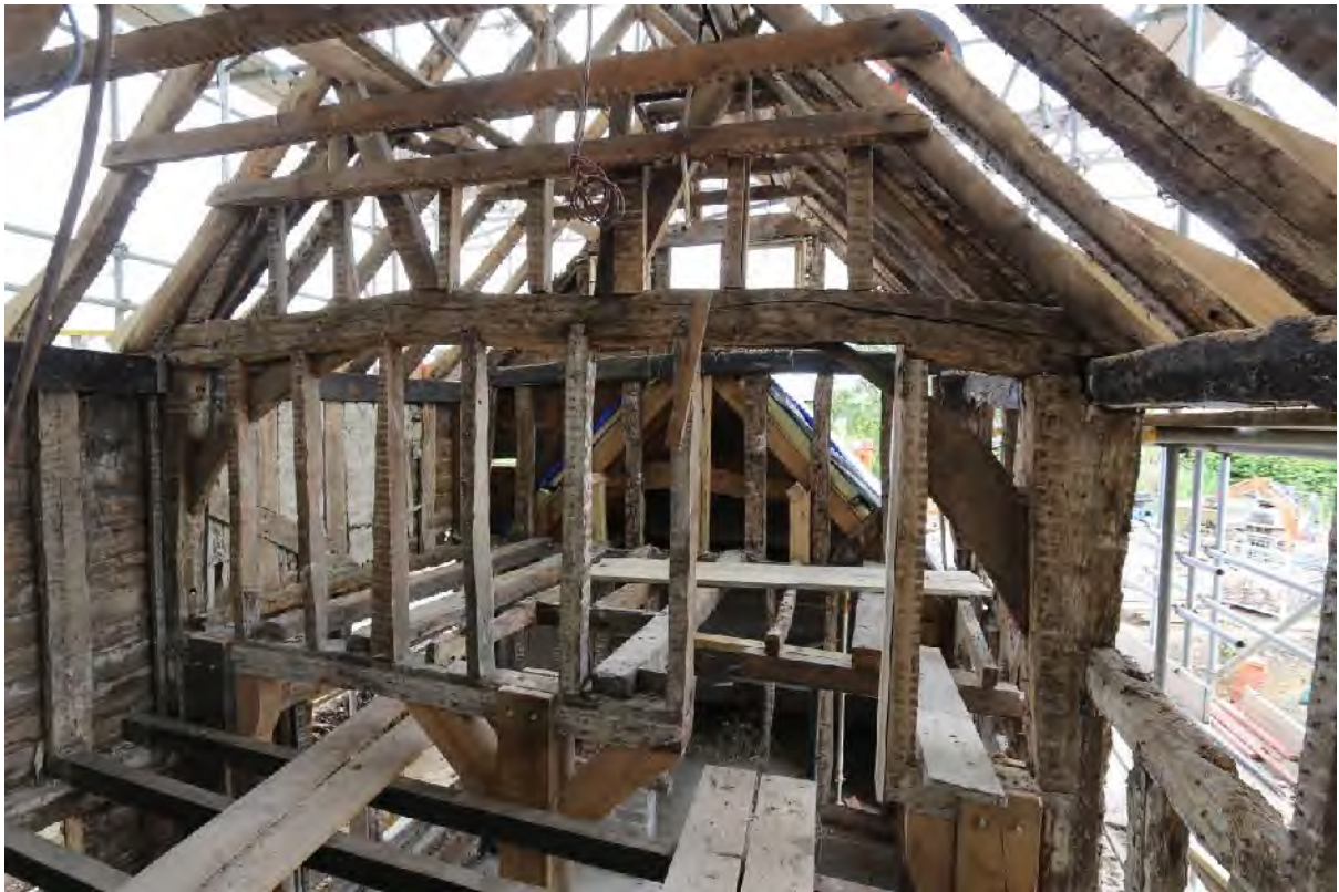
Plate 84 Northern wall of (F6), showing cut through transverse beam and arch braces
