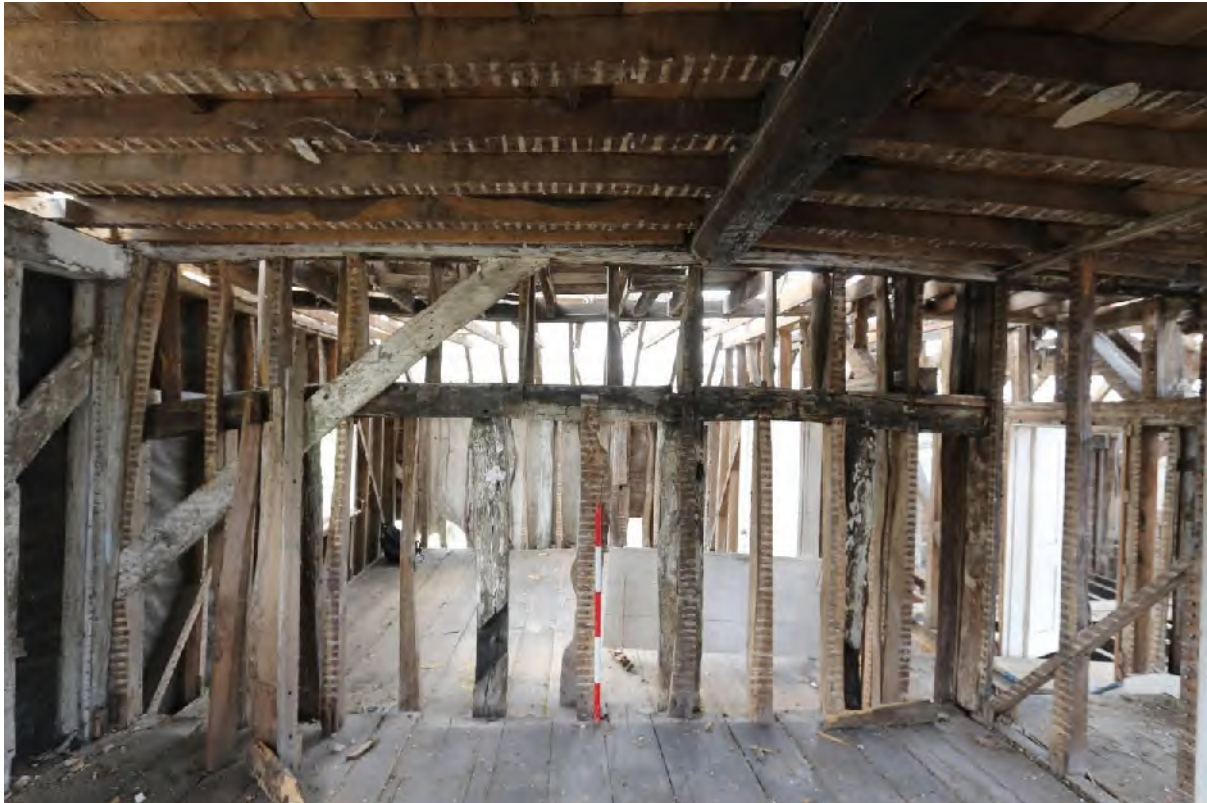
Plate 73 Eastern wall of (F1) showing empty trenches for tension braces, looking west from (F2)
