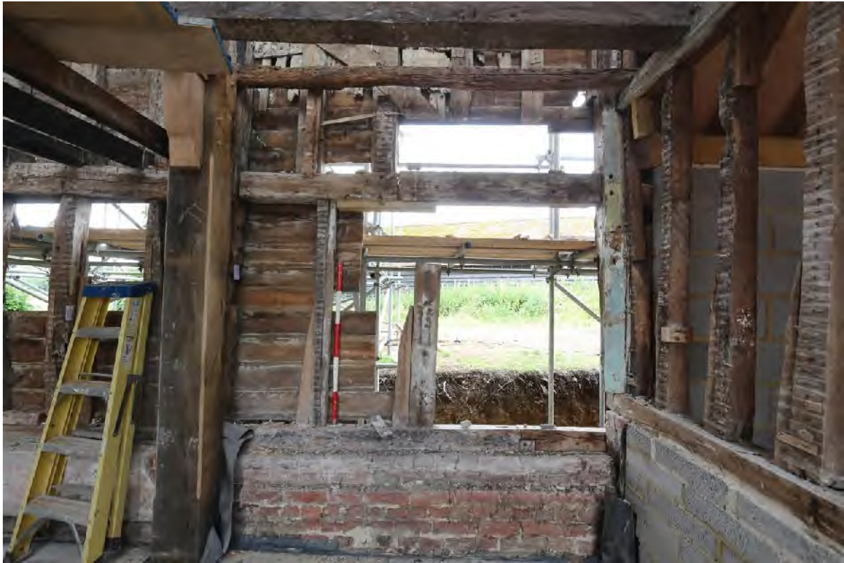
Plate 63 Western wall of (G4) showing cut away brace (upper register) and new section of mid rail.
