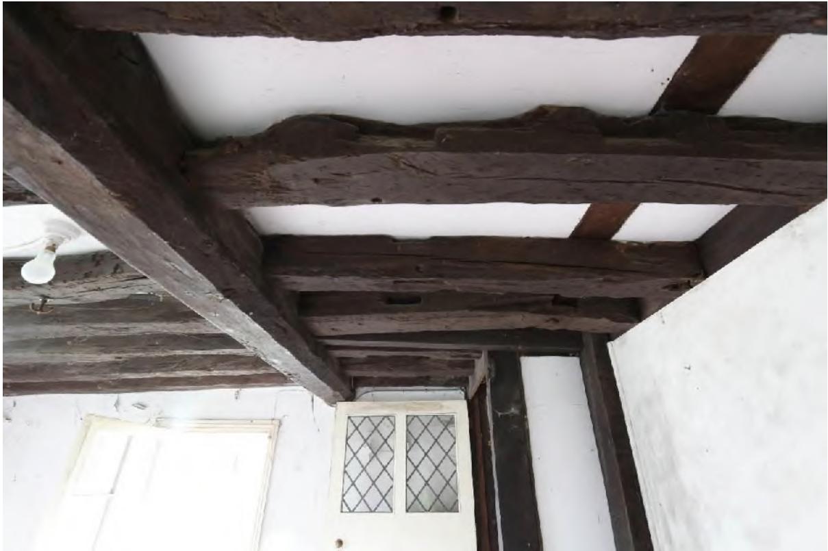
Plate 15 Detail of bridging beam and re-used timber for first floor joists (G1)
