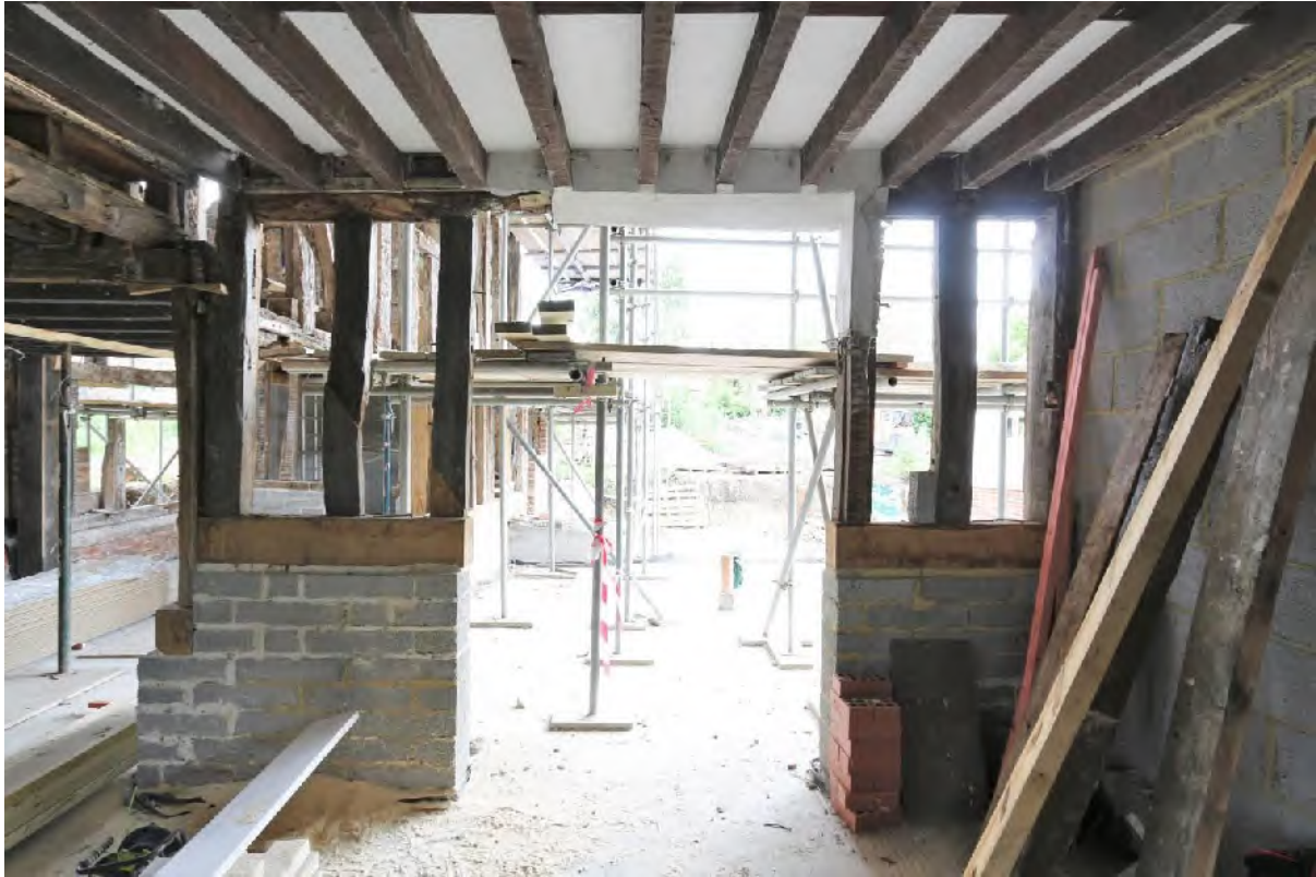
Plate 59 North wall of (G2) showing evidence for tension brace (left of opening)
