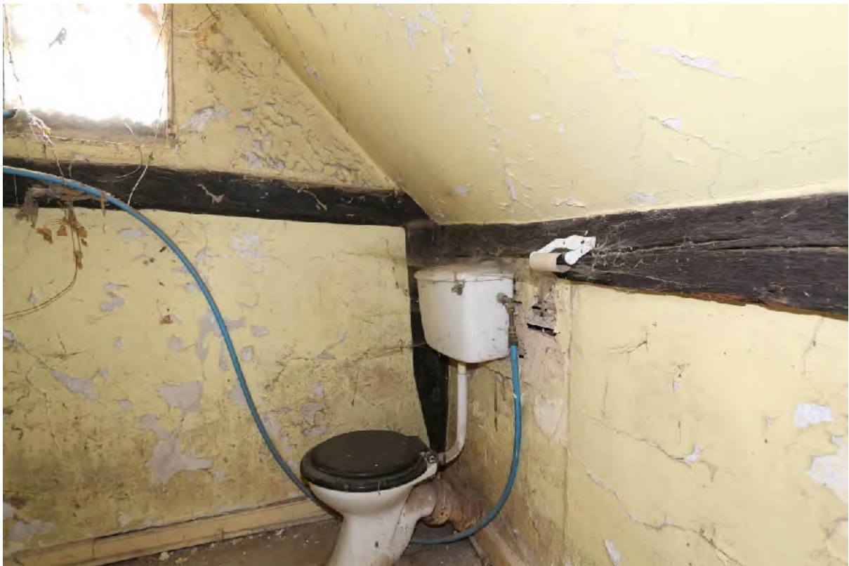
Plate 38 Bathroom (F7), showing wall plate, tie and jowled storey post, looking north-east
