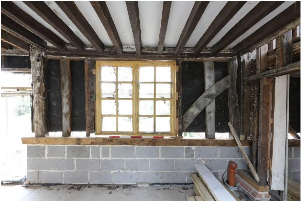
Plate 56 Southern wall to (G2) showing downward brace
