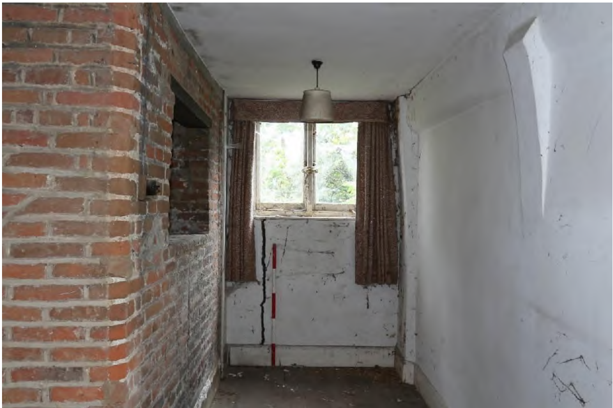
Plate 34 Bedroom (F2), detail of jowled posts (right) and structural crack in blocking wall
