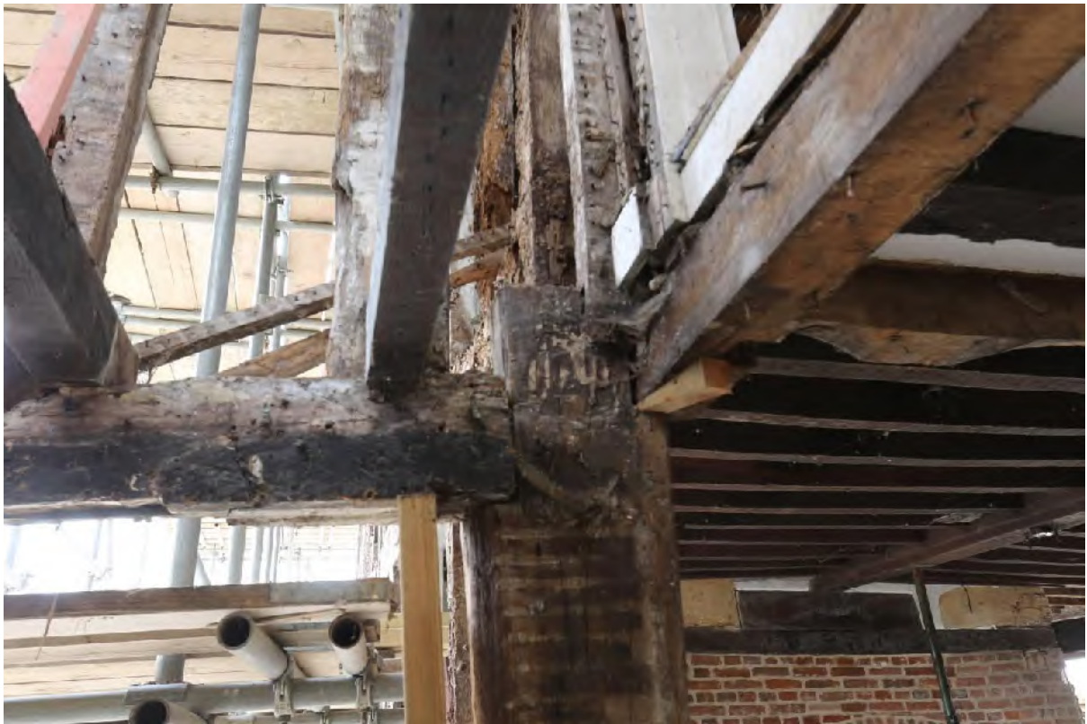
Plate 62 Post carrying the cut back mid rail and primary braced wall frame at first floor
