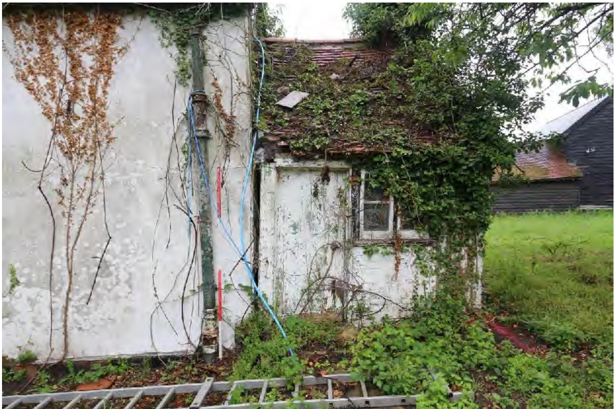
Plate 12 Small in-line extension pulling away from cross-wing
