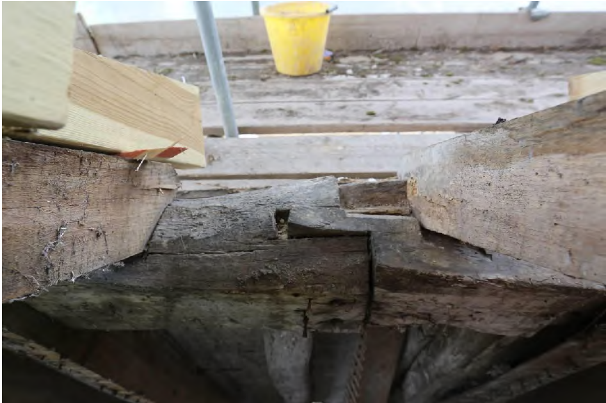
Plate 71 Face halved scarf joint in western top plate of (F1)
