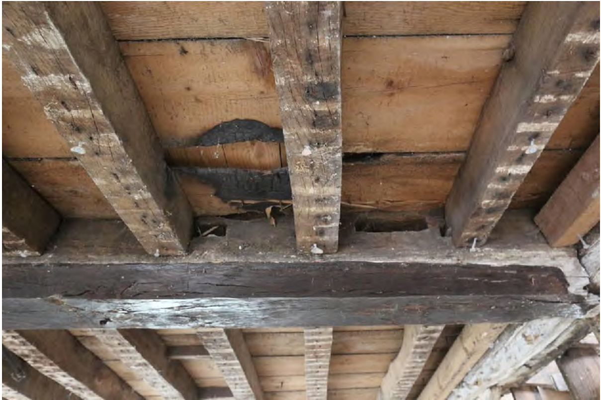
Plate 79 Empty mortices in re-used bridging beam (F2)
