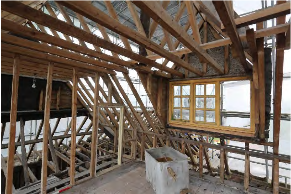
Plate 97 Post fire roof structure and dormer to attic room over (F1 and F2)
