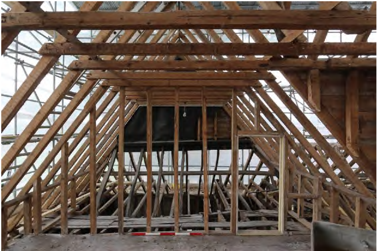
Plate 98 Post fire roof and stud wall in attic
