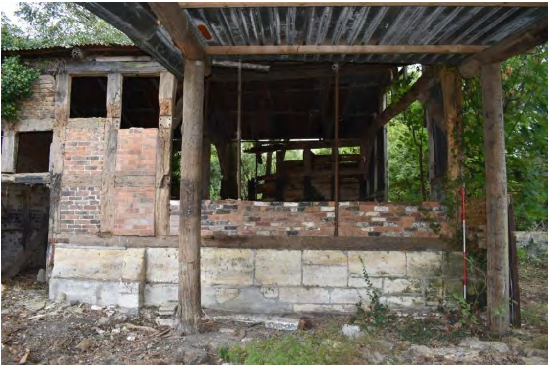
6 Area where timber framing has been replaced by iron poles and brickwork
