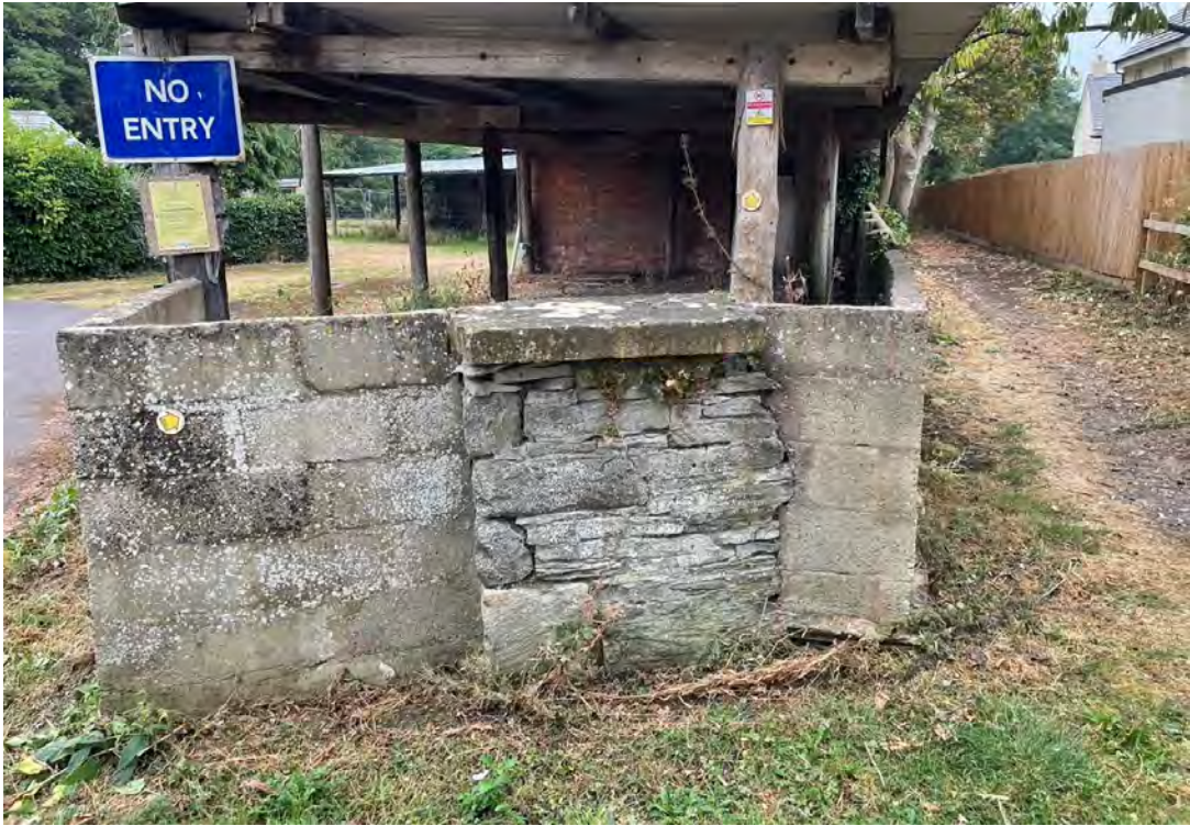
54 Section of stone walling of former building or boundary wall at north end of site, surrounded by breeze blocks of Building M, looking south
