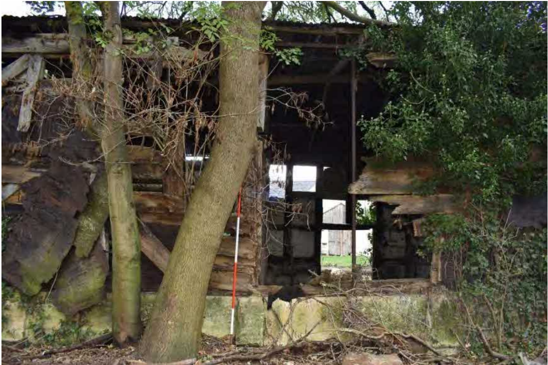
7 South-west side of the building with timber framing replaced by iron pile
