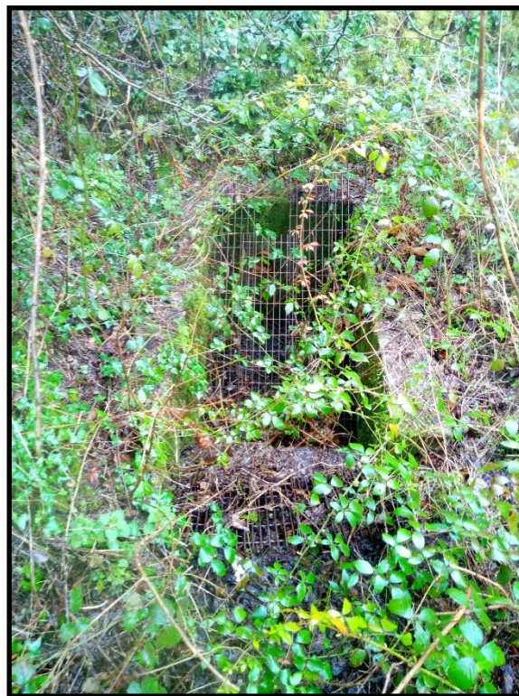
Photograph 10 – Photo of a leat or structure related to a water course. This was located in the southeast corner of the site. Please note extensive vegetation cover in this area limited the visual inspection.
