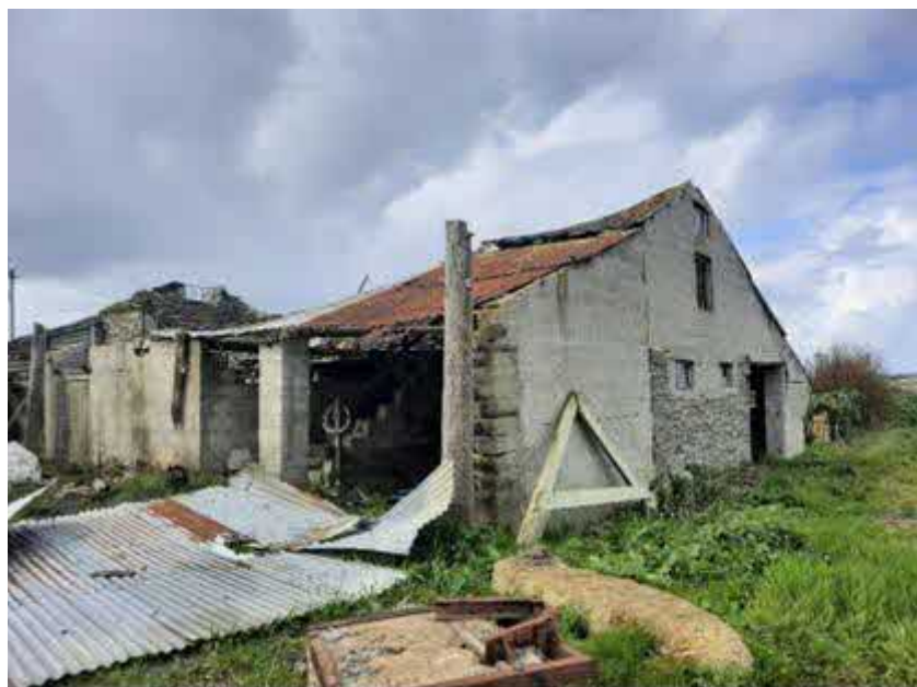
Figure 6: View of part of the block-built dilapidated section on the northeast elevations of Barn 2.
