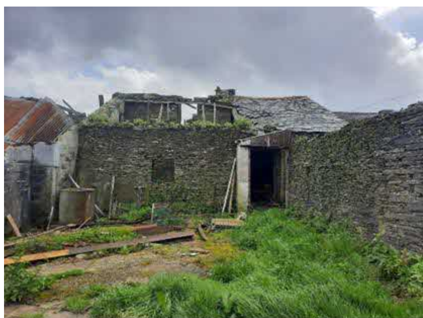
Figure 4: View of part of the stone-built section on the western elevation of Barn 2.
