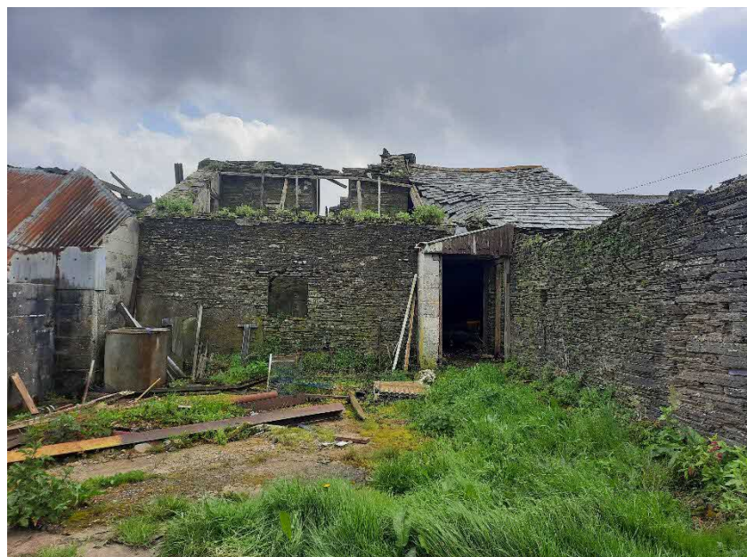
Figure 6: View of part of the stone-built section on the western elevation of Barn 2.
