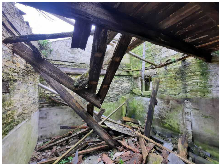
Figure 11: Internal view of part of the dilapidated stone-built section in Barn 2.
