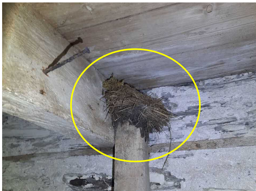
Figure 14: View of an old likely blackbird nest that has been repurposed by a tit species (yellow circle); located under the timber joists at the wall top within Barn 2.
