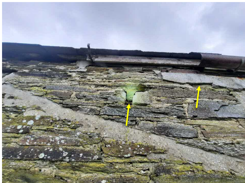
Figure 9: View of gaps within the stonework and beneath render (shown by the yellow arrows) on the western elevation of the stone-built part of Barn 2.
