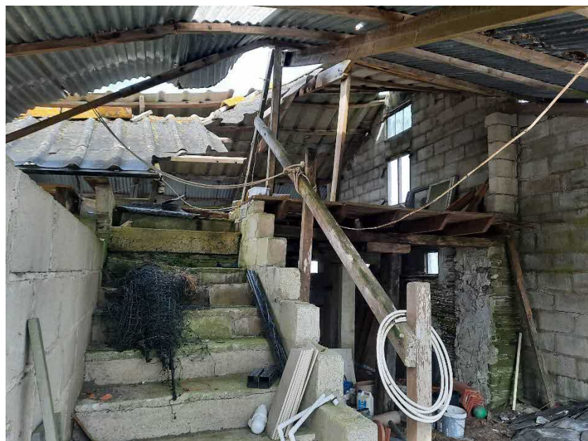
Figure 10: Internal view of part of the dilapidated block-built section in Barn 2.
