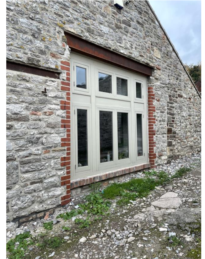
Window to the east elevation which has been constructed with a higher cill than approved to take account of existing adjacent ground levels.
