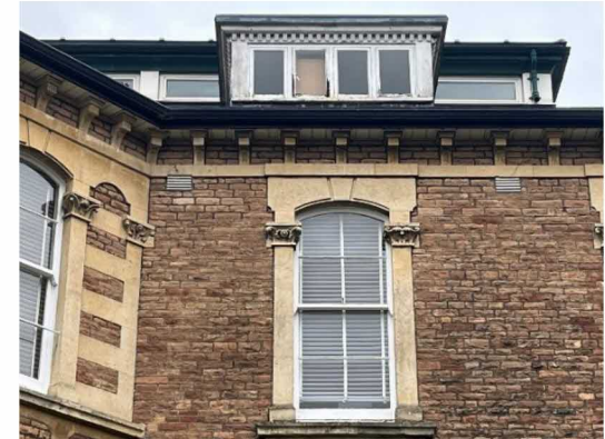
Photo 5. The eaves with stone corbels above which is a 20 th century dormer window. Behind this is the clerestory that was added c. 1998.
