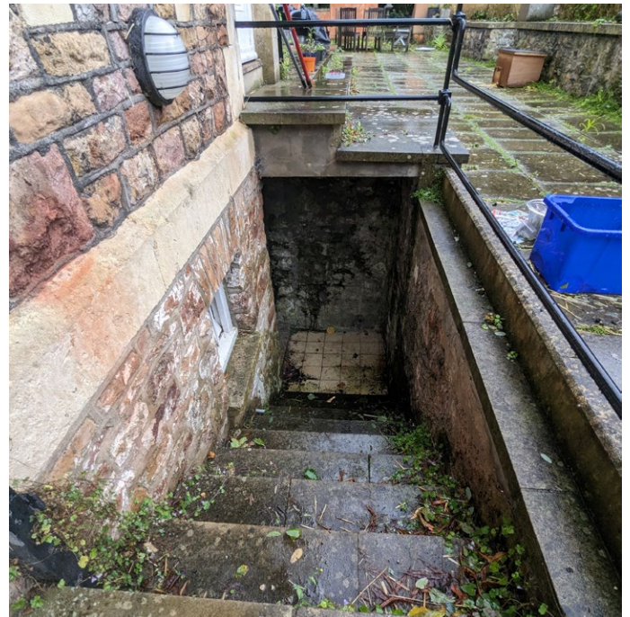
Existing steep and unsafe steps to lower ground floor at rear.
