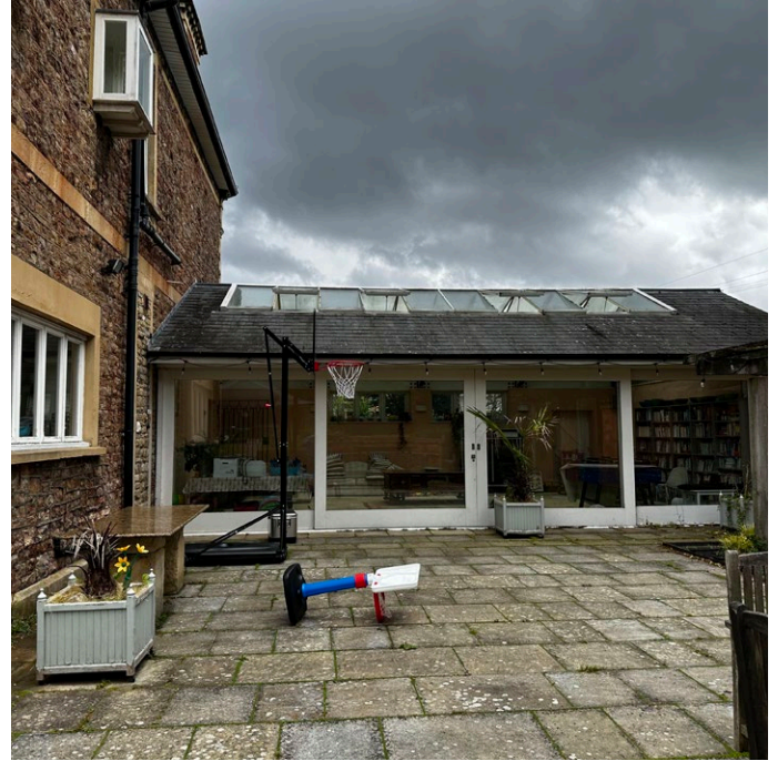
The existing extension from the rear. The structure is not weather-tight and the sliding doors are failing.
