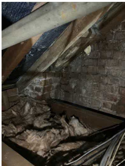
Figure 15 - Evidence of Moisture Ingress to Roof Void
