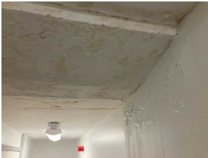
Figure 13 - Internal Water Ingress
