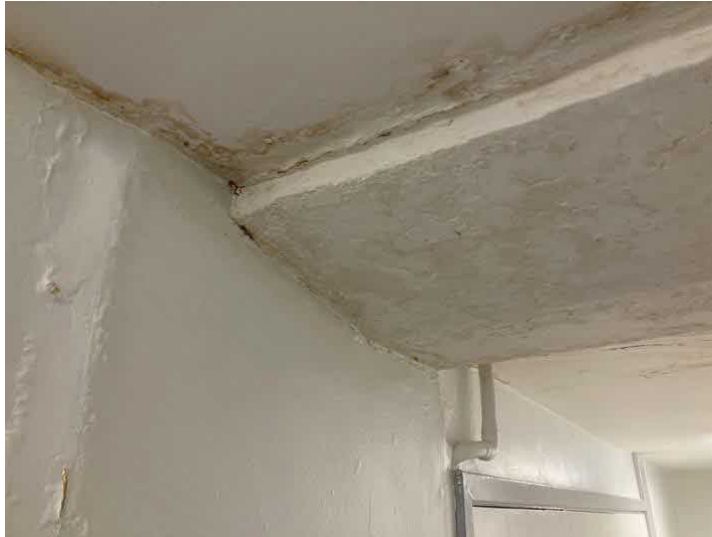
Figure 12 - Internal Water Ingress
