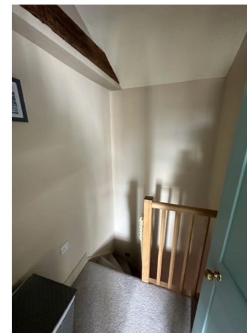
View from second floor landing looking toward position of proposed new window.
