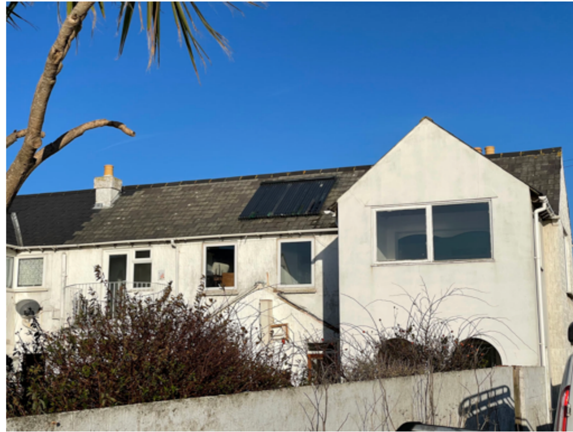
2. View of existing roof mounted solar thermal panel viewed from Wellington Parade
