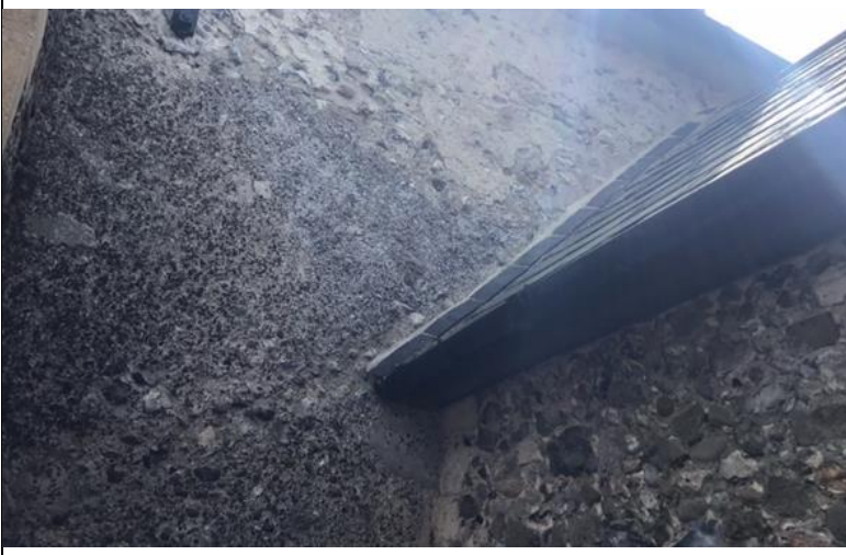
above, former lean-to prior to construction of vestry extension, below victorian wall abutment to nave
