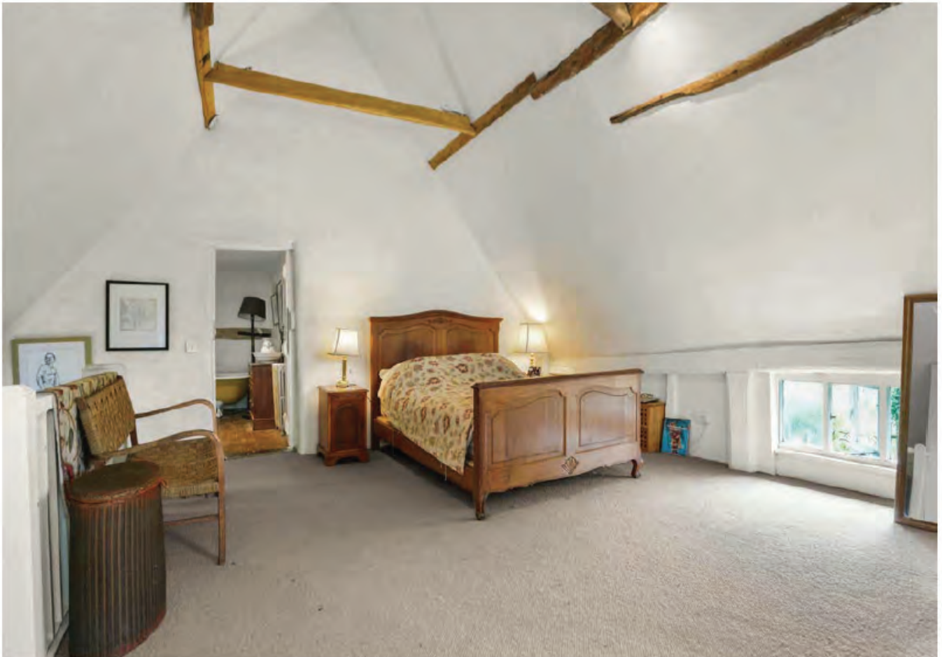
Pic 8 Repaired roof collar and purlins, final lime plaster over savolit board. Sheeps wool insulation.
