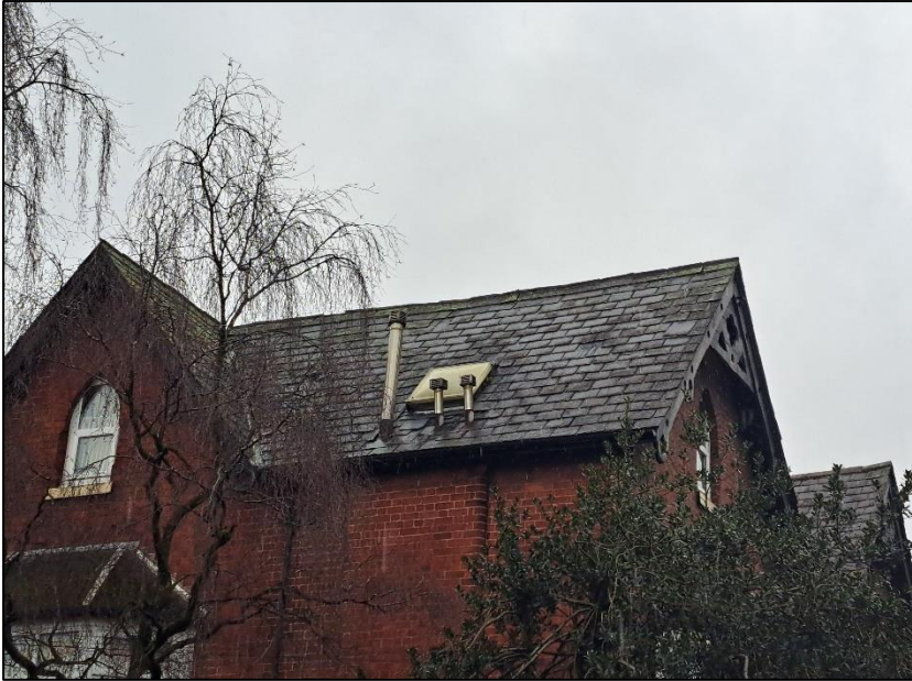
Photograph 2: Showing slipped tiles on roof facing south.
