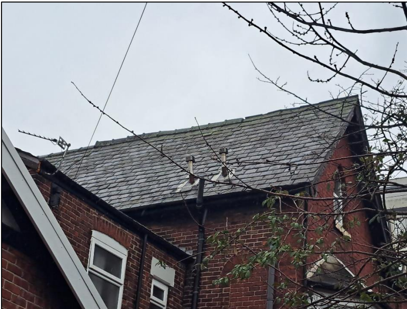
Photograph 5: Showing gaps between ridge tiles.
