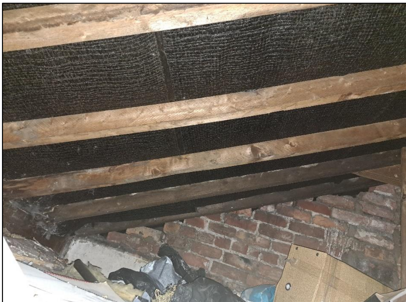
Photograph 7: Showing gaps between rafter and wall
