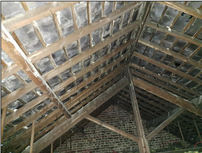
Photograph 9: Showing unlined roof void.
