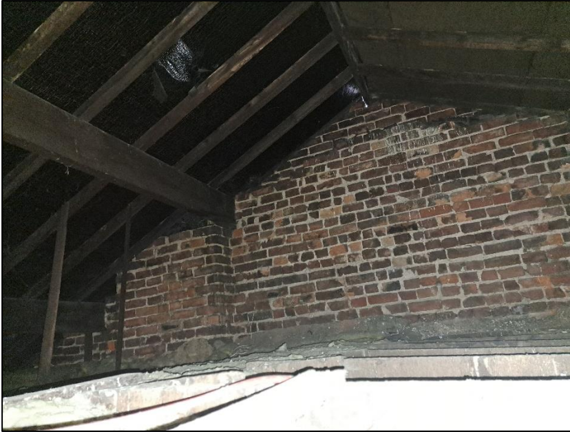
Photograph 8: Showing daylight visible at the gable apex.
