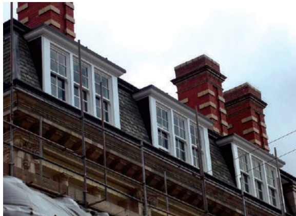
Dormer windows on part of the Railway Offices, Altrincham, part of a 400-window restoration
