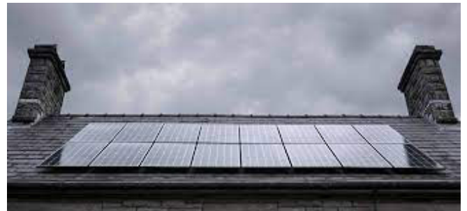
Above: Example of photovoltaic panels
