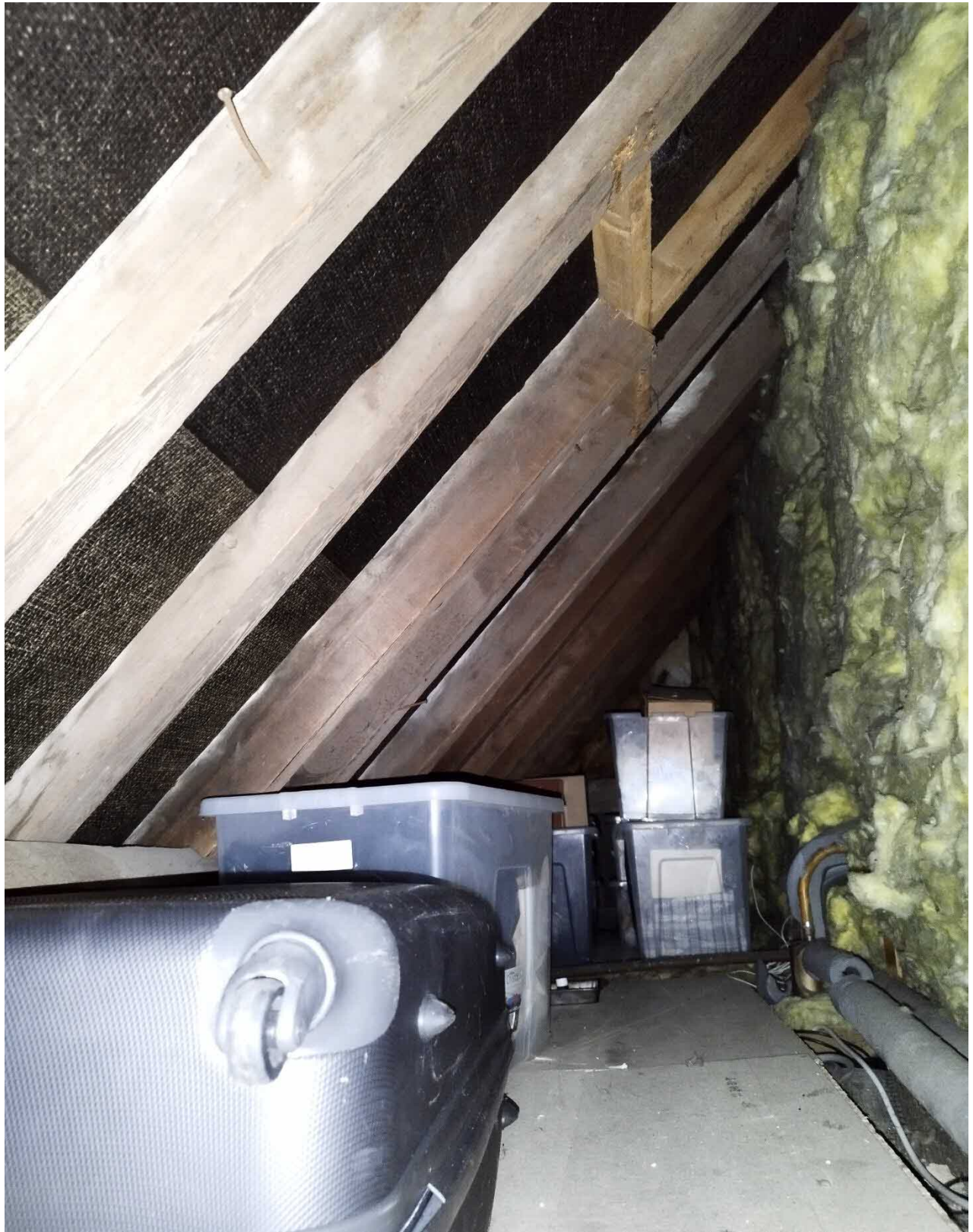
Internal View showing the existing 'modern' roof structure above the rear Kitchen extension. (taken within the roof void at first-floor level above the existing kitchen).
