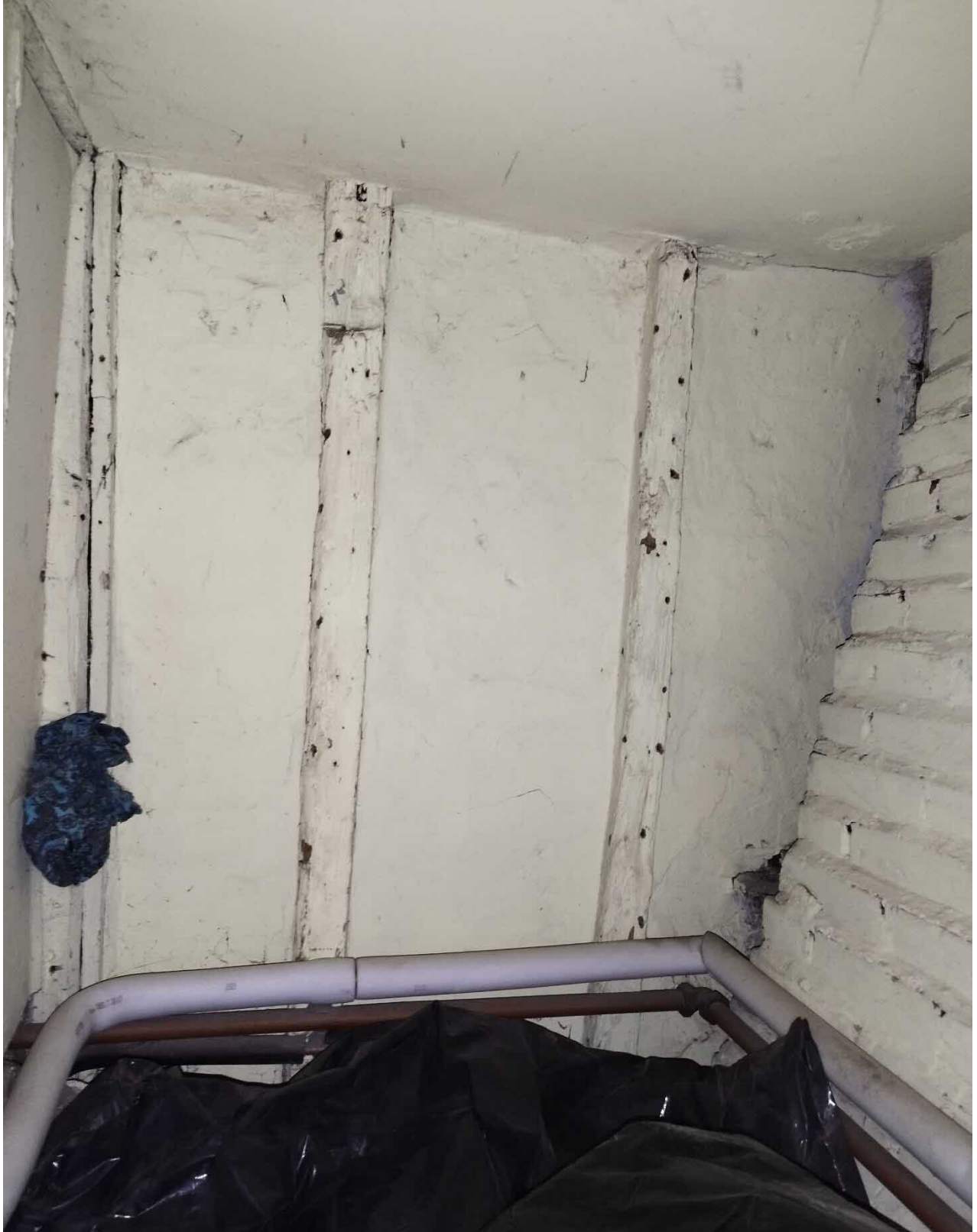
Internal View showing the area of wall where the new door from the bedroom to the new en-suite is to be inserted (taken from the existing first-floor cupboard).
