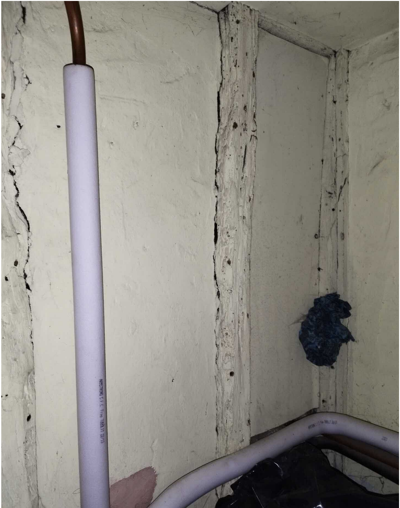
Internal View showing the area of wall where the new opening within the new en-suite is to be formed (taken from the existing first-floor cupboard).
