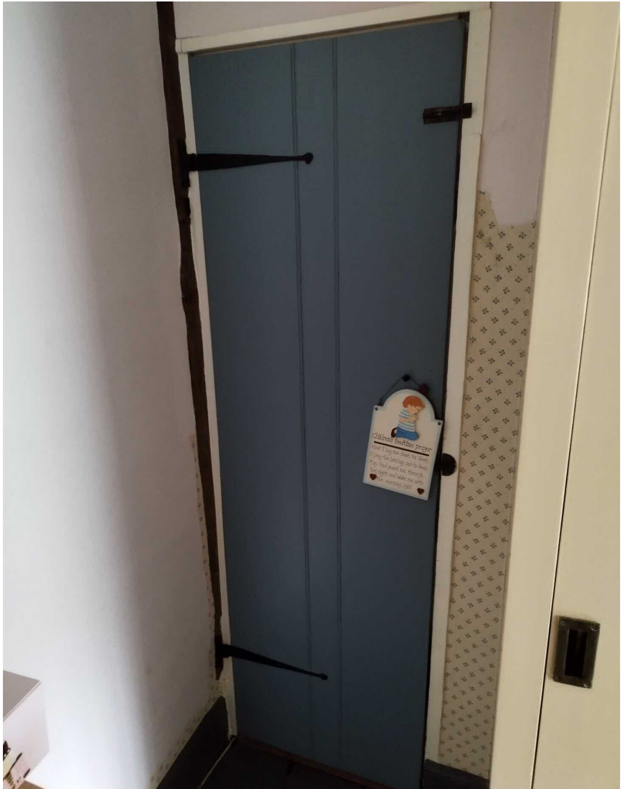
Internal View showing the existing doorway to be infilled to form the new en-suite is (taken from the existing first-floor bedroom).
