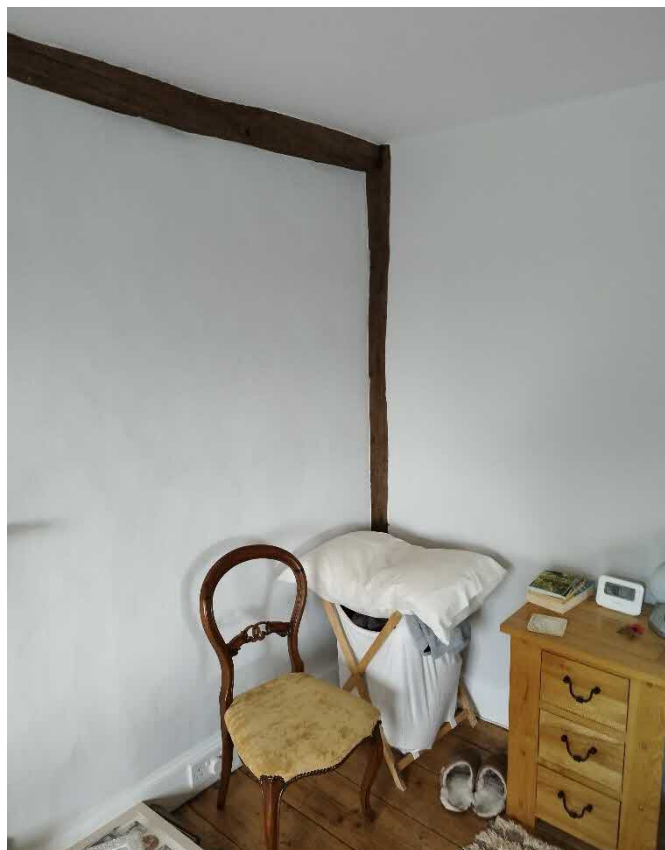
Internal View showing the area of wall where the new door from the bedroom to the new en-suite is to be inserted (taken from the existing first-floor Bedroom).
