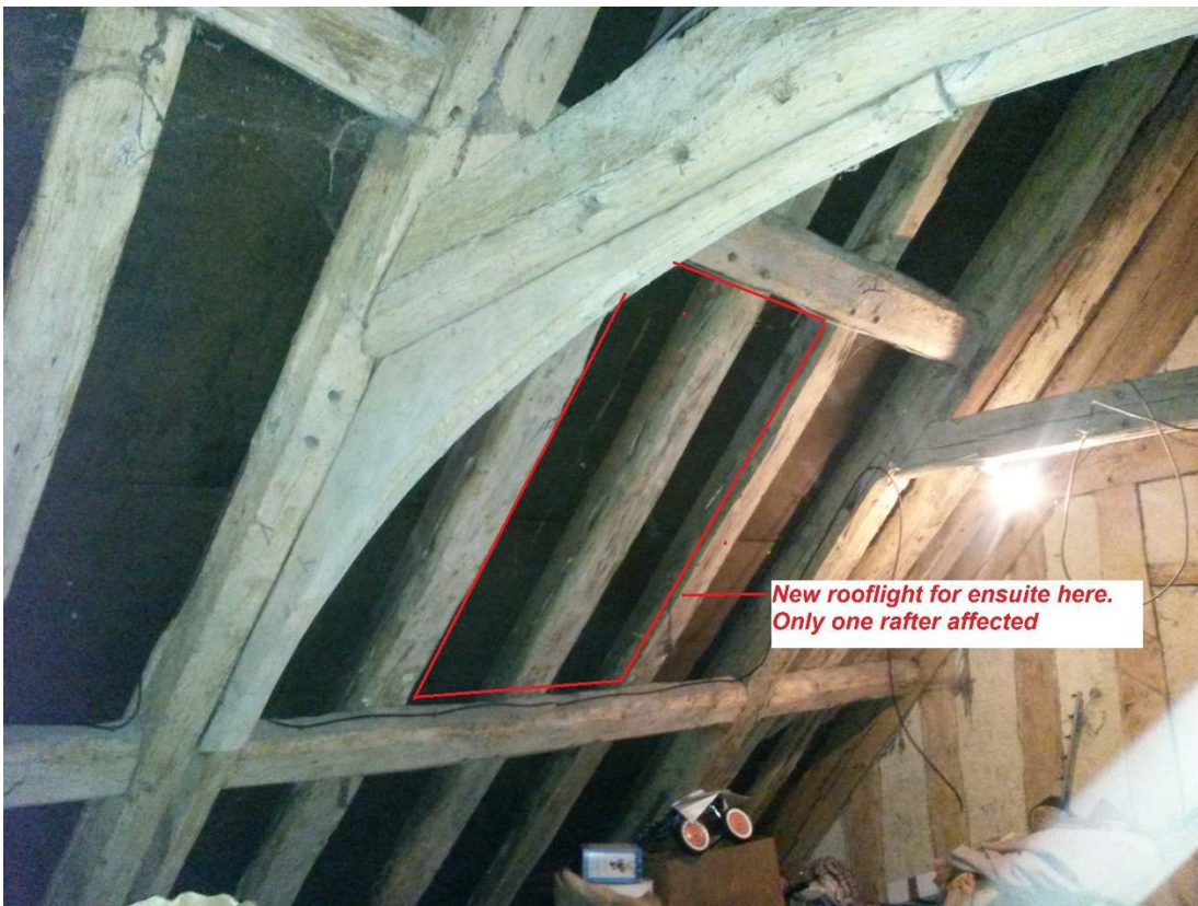
Existing roof with new rooflight for ensuite. 2 other new rooflights serving new attic bedroom positioned similarly to affect only one rafter each.
