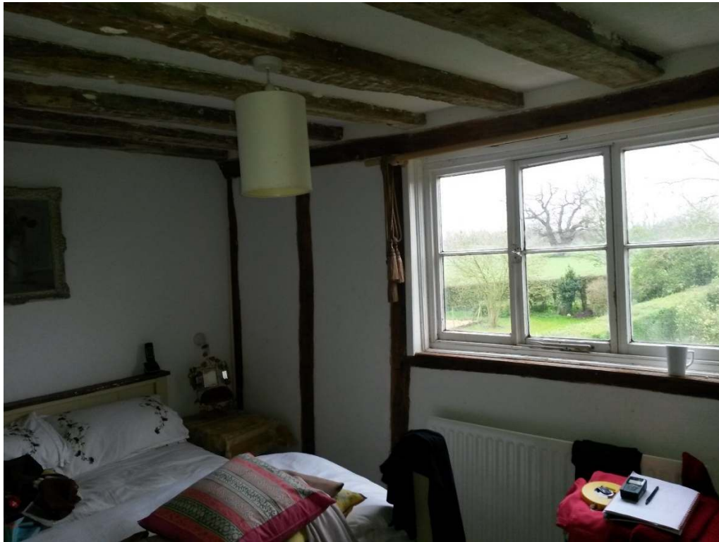
The first-floor window that will need replacement to achieve means of escape requirements following discussion with Building Control
