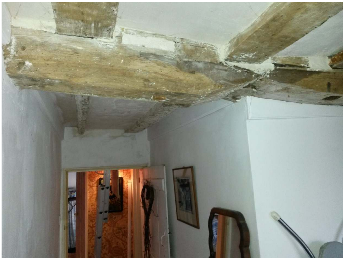
First floor showing existing door at landing level that will be upgraded to be fire resistant. ARCHITECTS TWO LTD FEBRUARY 2024
