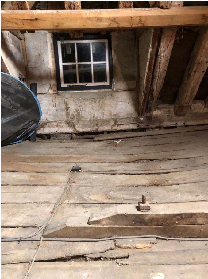
Earlier repair to weakened spine beam to be replaced with suitable steel fitch plates to engineer's design.
