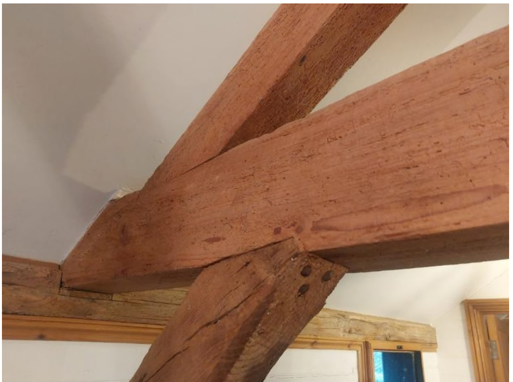
Figure 9 Detail of the joint between the tie beam, brace and principal rafter showing the lack of pegged joints, the brace being notched and nailed to the tie beam.
