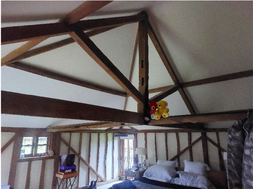
Figure 8 The bedroom at the east end of the upper floor showing the studwork to the walls and king post roof truss.
