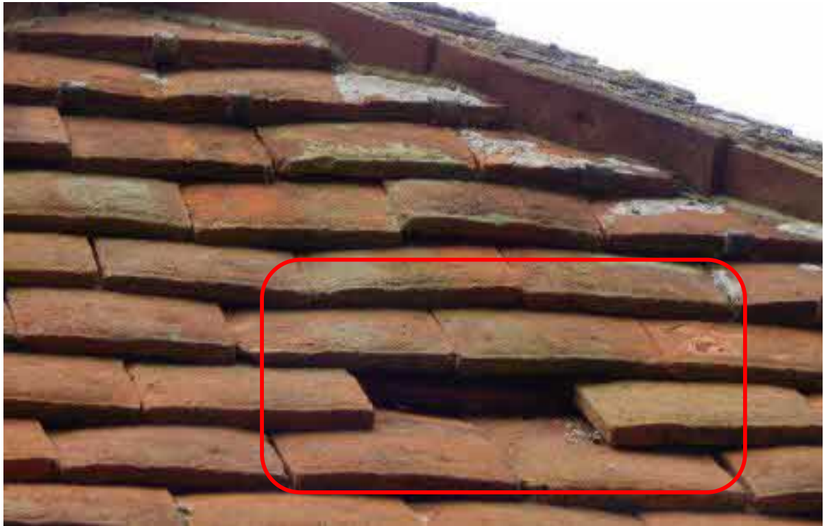
Image 4 – B1 – Gaps observed within the South facing vertical hanging tiles
