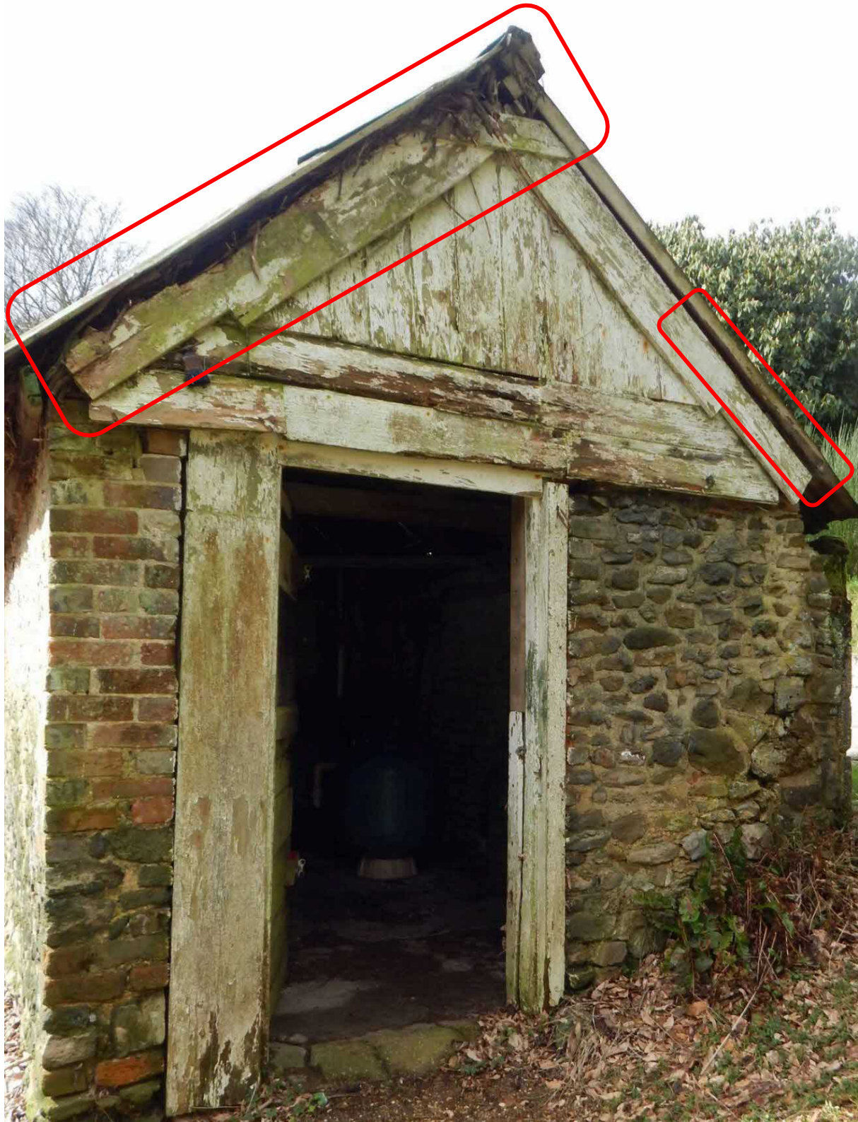
Image 12 – B2 – Front elevation of the structure offering further gaps between the roof coverings and timber fabrics below
