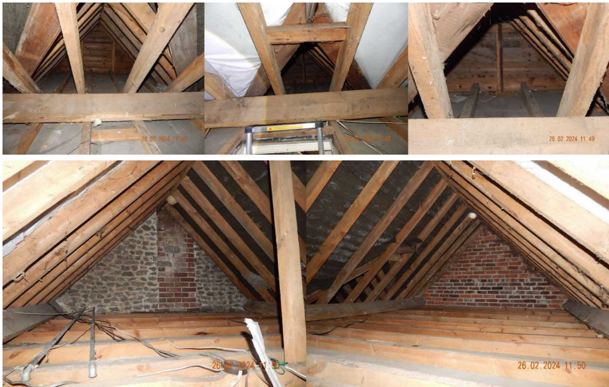
Image 9 – B1 – Internal view from within the main upper roof coverings of the property
