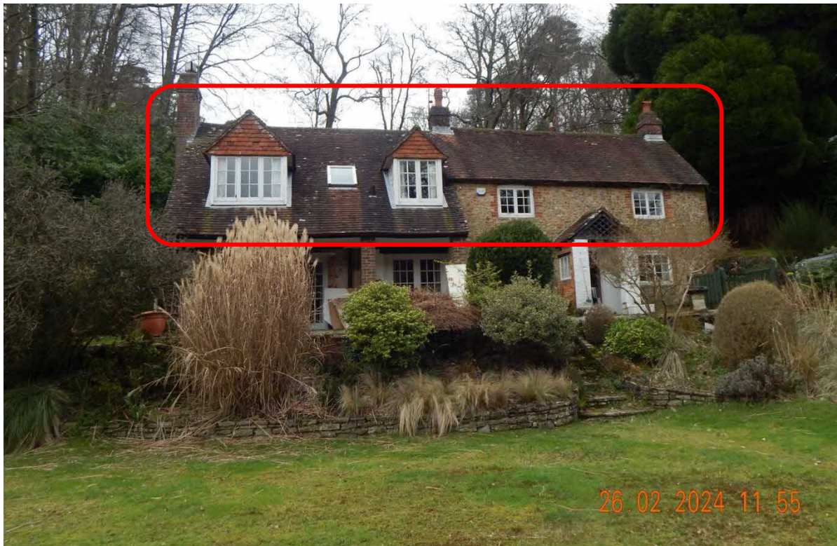
Image 2 – B1 – South facing elevation of the structure which has demonstrated a moderate level of gaps of accessible proportions to offer value to bats
