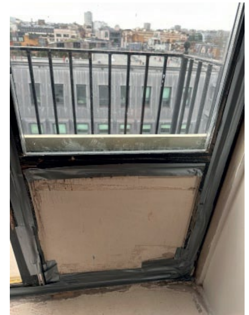
The windowpane was cut to allow for ducting. It has been boarded to prevent rain coming in.
