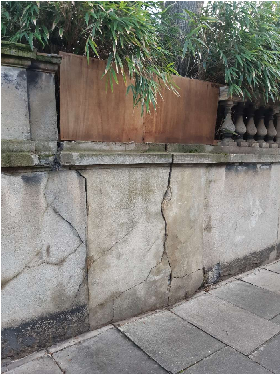
Substantial damage to boundary wall by T1
