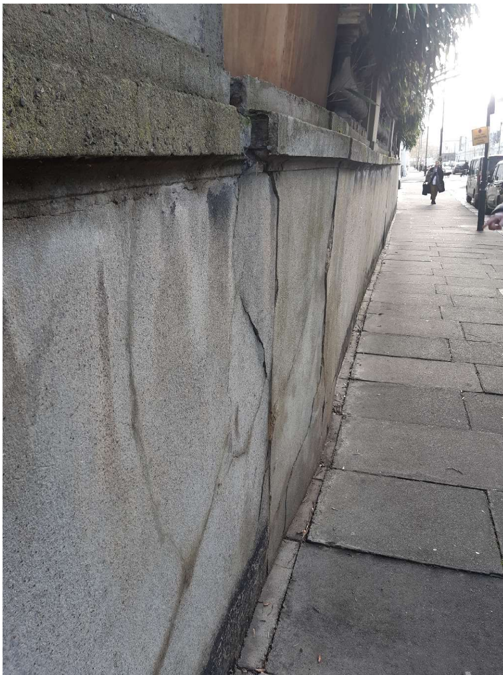
Damage to boundary wall (clearly pushed out of alignment)
