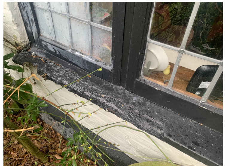
external view - damaged cill
