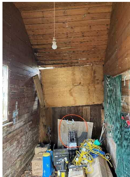
Figure 31 – View to north wall, note temporary ply repair at top of wall
