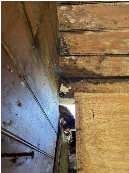
Figure 33 – North west corner, timber decay due to hole in roof
