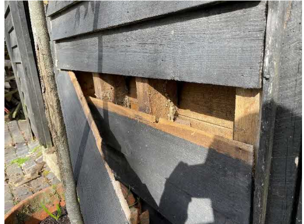
Figure 29 – Loose board between doors, no membrane
