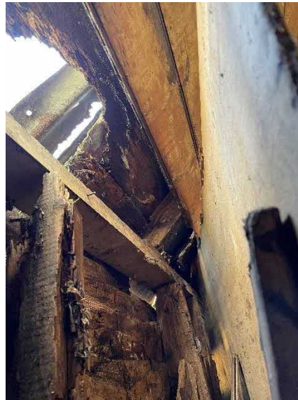
Figure 34 – Boards above rafters visible
