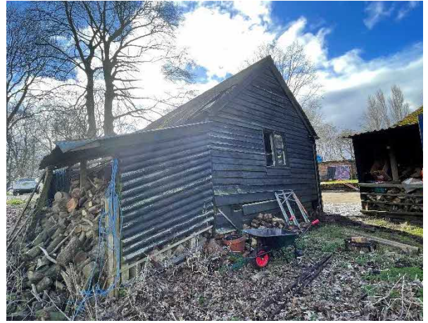
Figure 4 - West elevation of stable with lean to log store to left hand side
