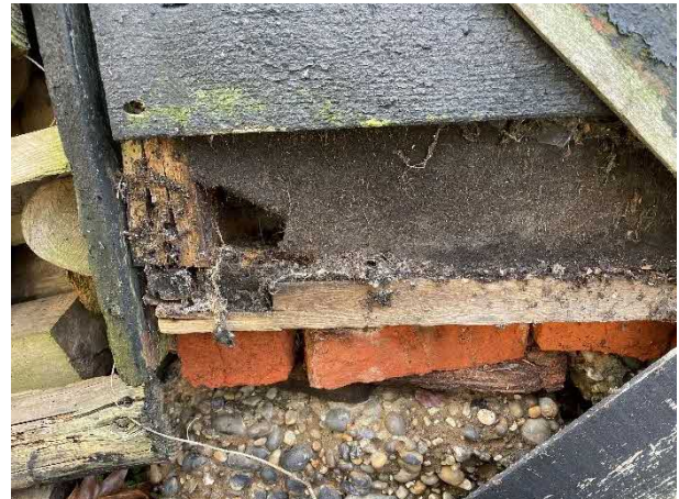
Figure 11 - Felt membrane ripped and sole plate decayed. Loose bricks with ply packing
