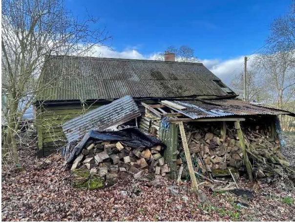
Figure 14 – Joists beneath floor boards. Damp and rot visible to boards and joists
