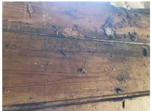
Figure 45 – Beetle attack to timber panelling
