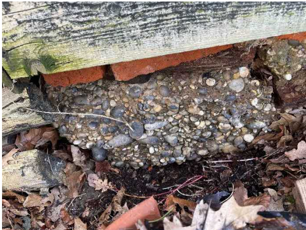
Figure 10 - North end of west gable, crack in slab 500mm from end loose bricks
