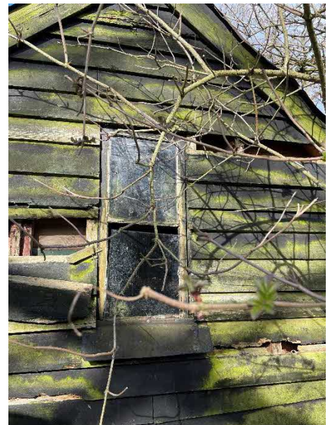
Figure 20 – Loose boards around window, with lower glazing slipped down
