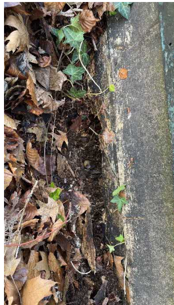
Figure 19 - Rotten boards at low level behind leaf litter and soil
