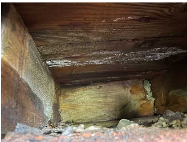
Figure 12 – Joists beneath floor boards. Damp and rot visible to boards and joists
