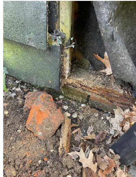
Figure 6 - Ripped felt membrane behind loose weatherboarding, decay to timber sole plate
