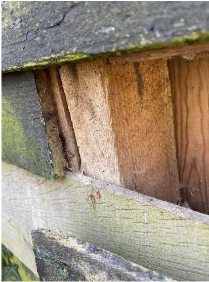
Figure 21 – Exposed stud with beetle attack in east elevation
