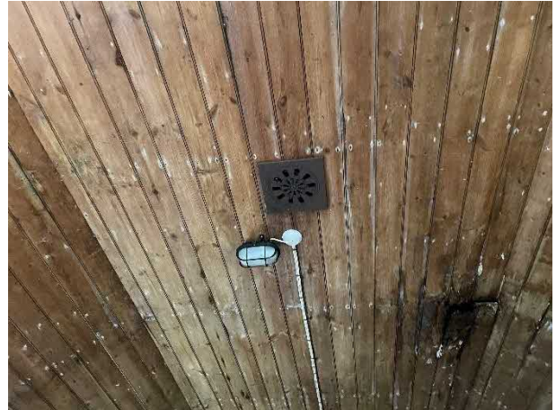
Figure 43 – Ceiling vent, water damage to right hand side
