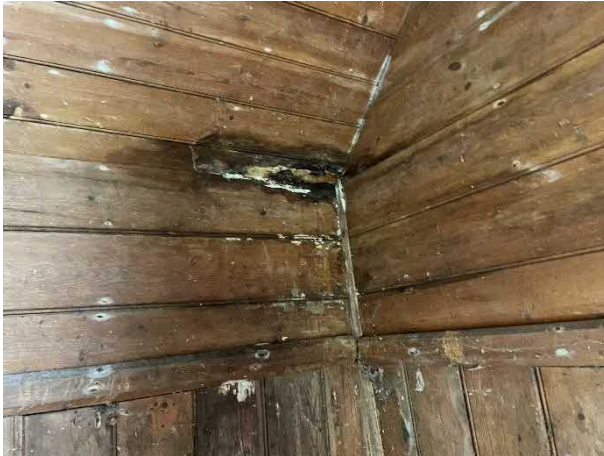
Figure 42 – Ingress of water and timber decay north east corner eaves level
