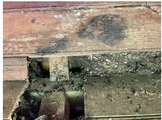
Figure 37 – Roof insulation and upper boards visible, beetle attack to inner boards
