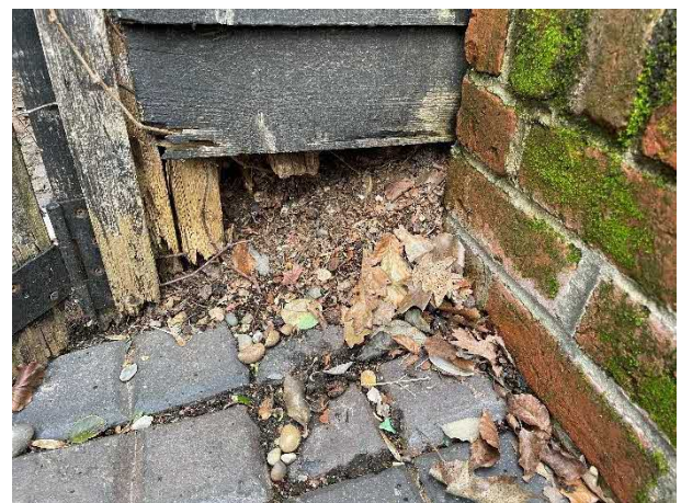
Figure 27 – Missing bottom board and decayed studs to right of east door
