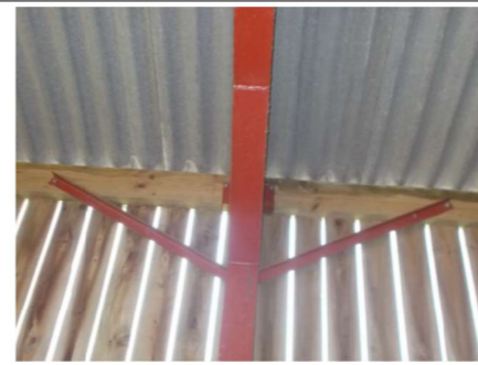
Typical - Longitudinal stability currently provided by lightweight steel bracing. Inadequate for conversion; detail elevations in such a way as to provide frame stiffness.
