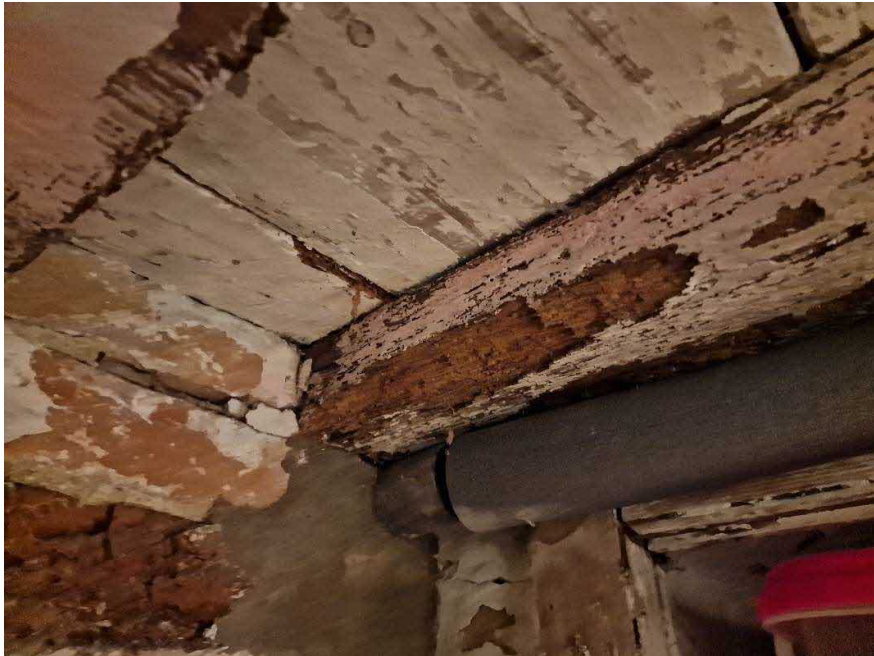
Image 1 – Rotten timber to basement ceiling
