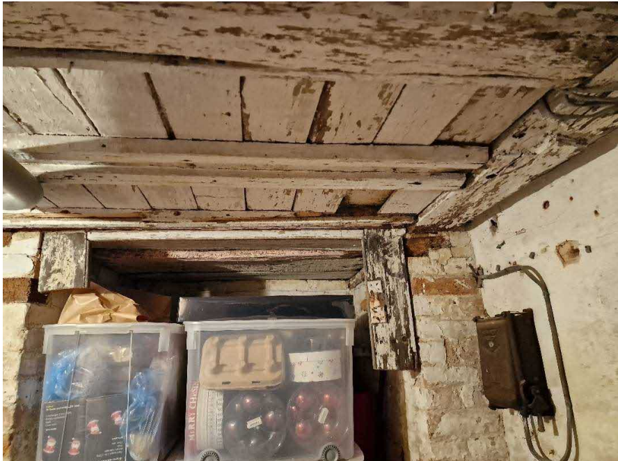
Image 2 – More basement ceiling joists which may require replacement
