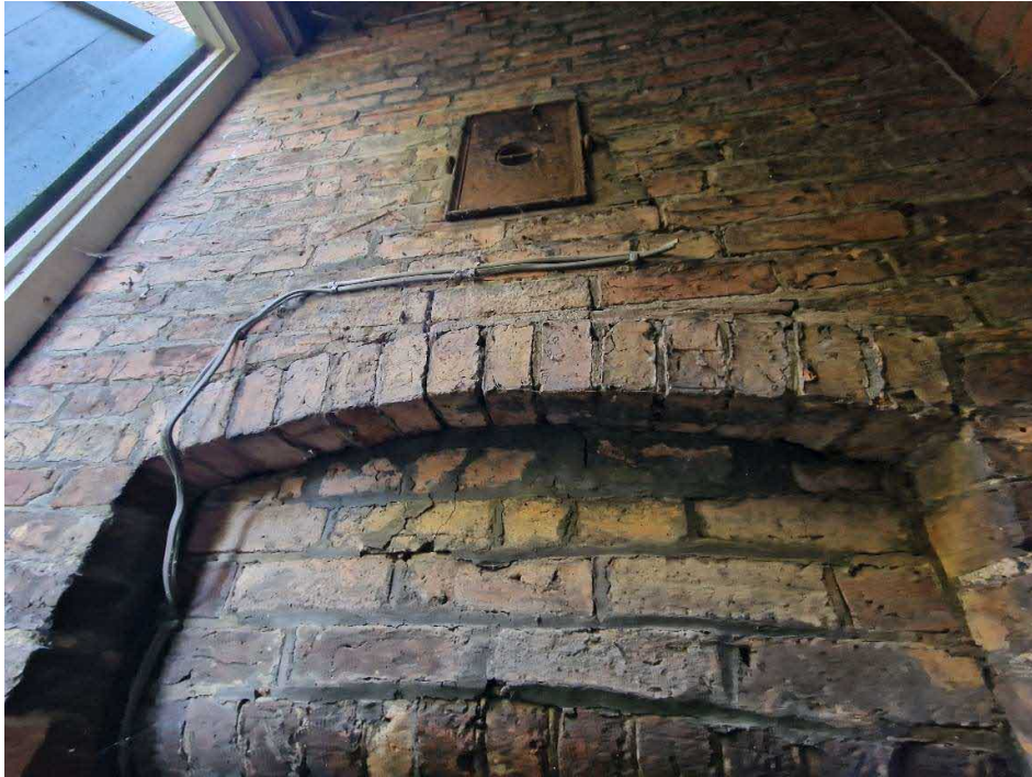
Image 3—Minor crack to brick arch lintel over basement door
