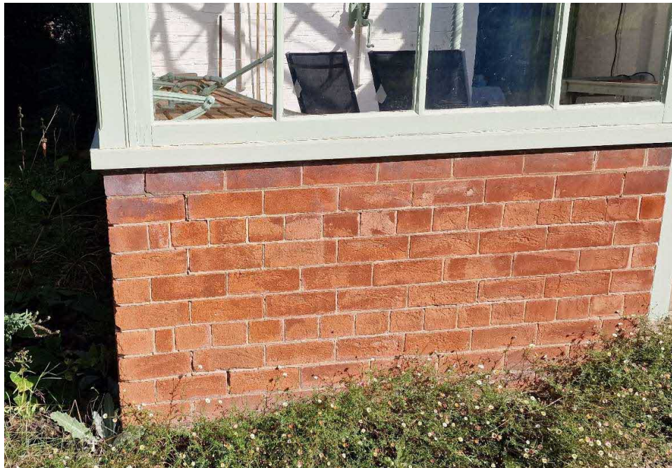
Image 4—Cracking to conservatory wall (left side)
