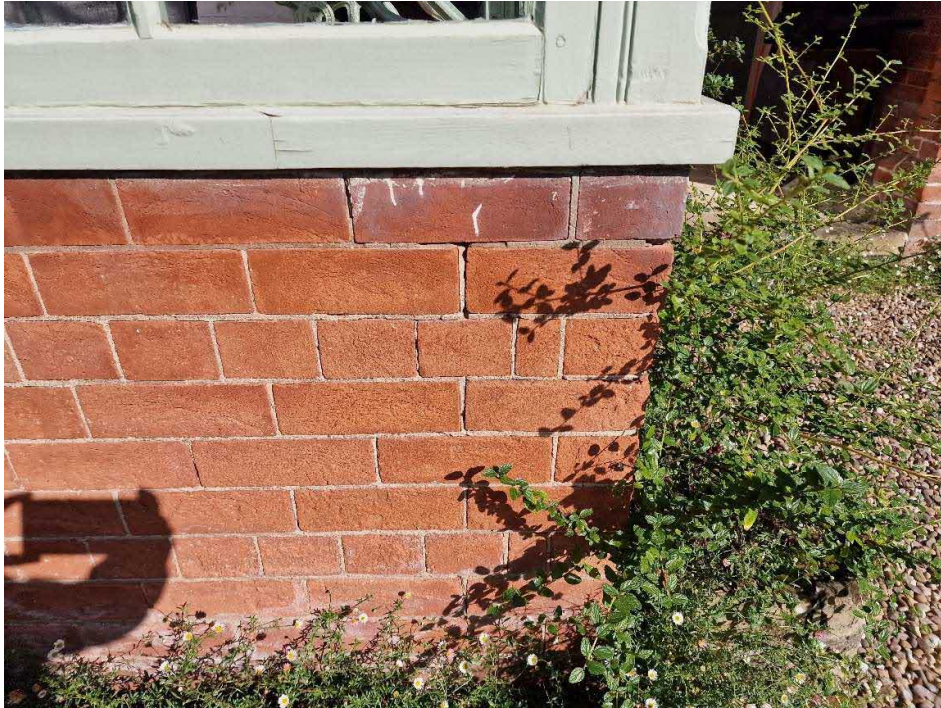
Image 5 – Cracking to conservatory wall (right side)
