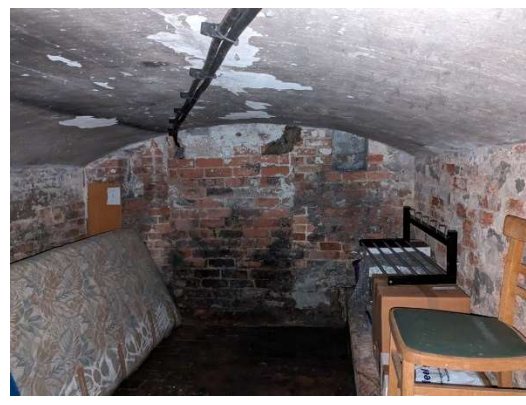
Internal view of small cellar. No obvious access points and well-sealed. No evidence of bats.
