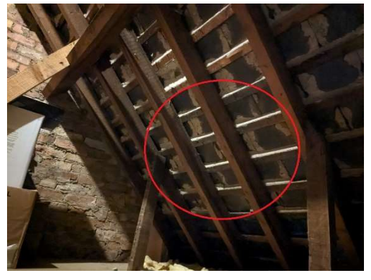
Internal roof void. Underside of slate roof at location of proposed roof vent. No potential access points or evidence of bats in this void.
