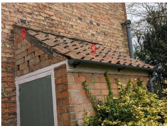
Cellar access door. Tiles along wall to be replaced. Shallow crevices unsuitable as PRFs.
