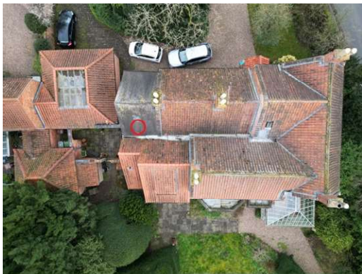
Location of proposed slate vent (marked in red). No PRFs noted and tiles sealed with mortar underneath.
