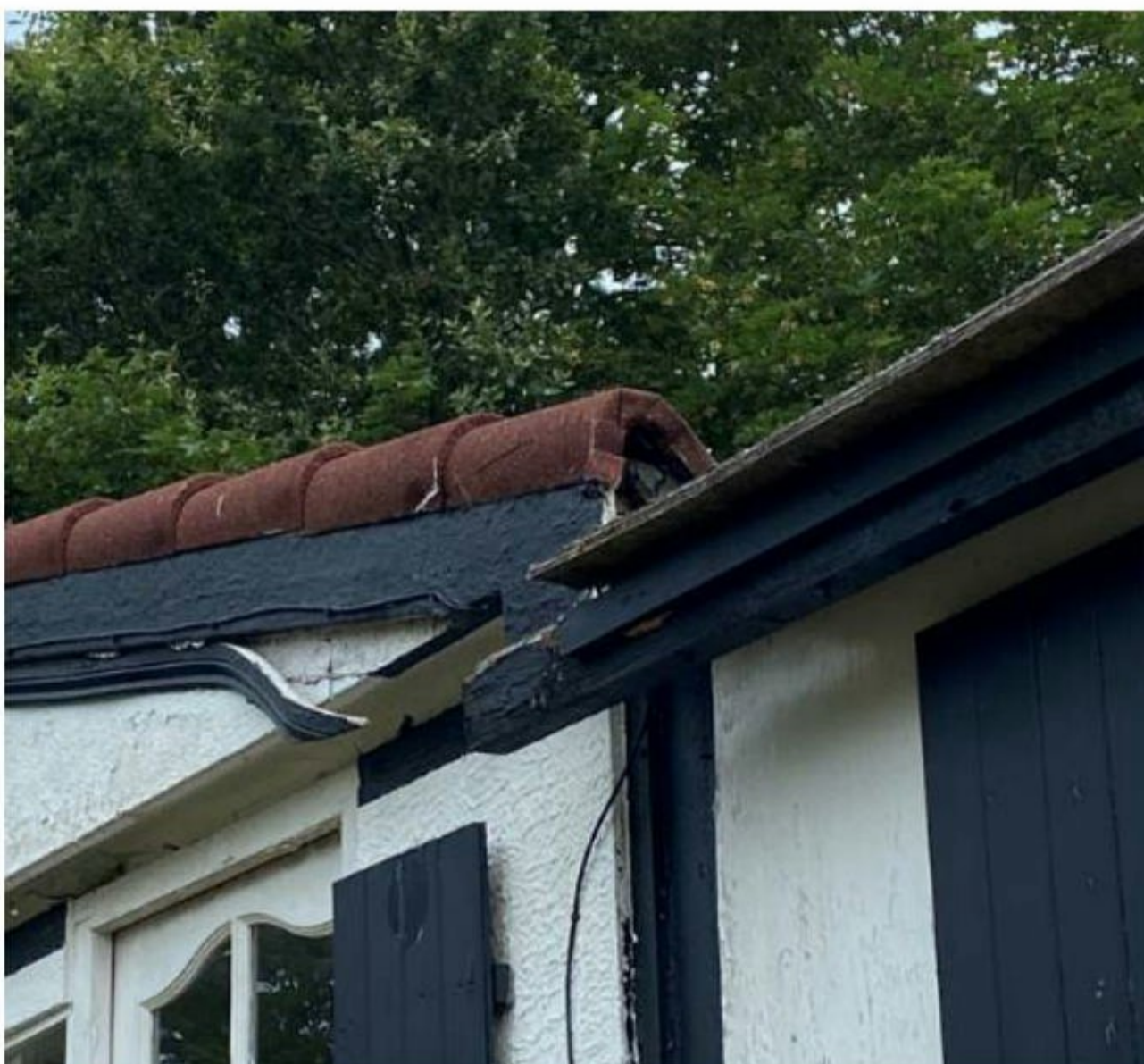
Photo 5: Close up of potential bat access point on the south-eastern corner of the pitched roof.
