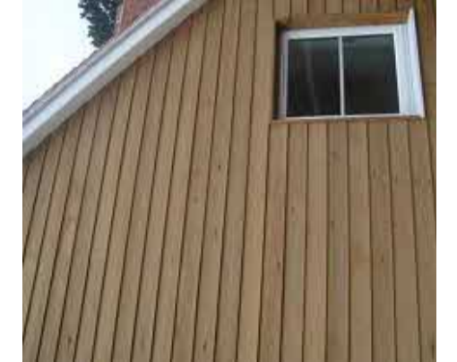
Natural coloured composite timber cladding to gables walls at first floor level
