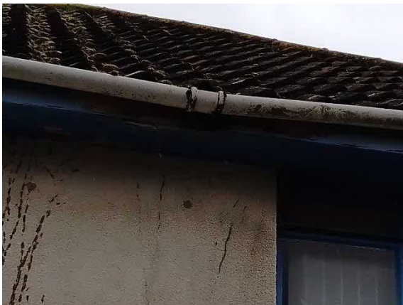
Photograph 3 – View of the hole in soffit beneath guttering.
