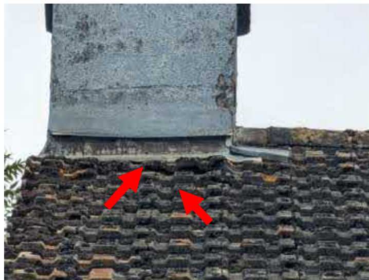
Photo 4. Showing the gaps between a number of roof tiles and the leadwork around the chimney
