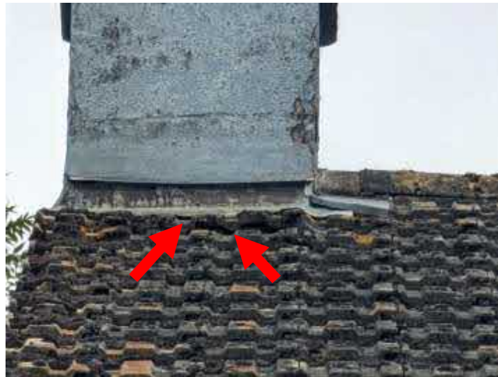
Photo 4. Showing the gaps between a number of roof tiles and the leadwork around the chimney
