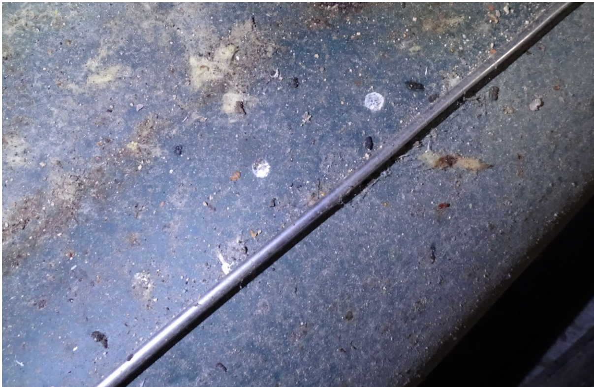
Image 22 – B1 – B1 – Internal evidence of bat droppings observed within the ground floor areas of the structure confirming activity from bats
