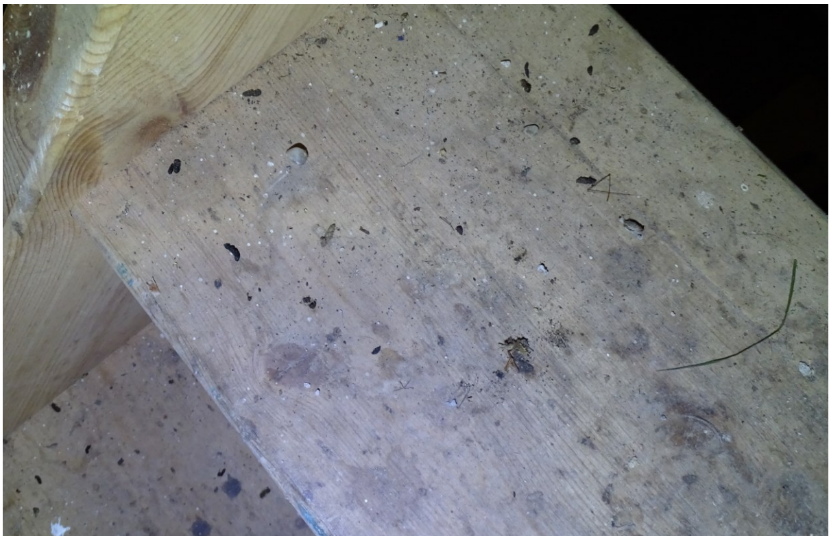
Image 21 – B1 – Internal evidence of bat droppings observed within the ground floor areas of the structure confirming activity from bats
