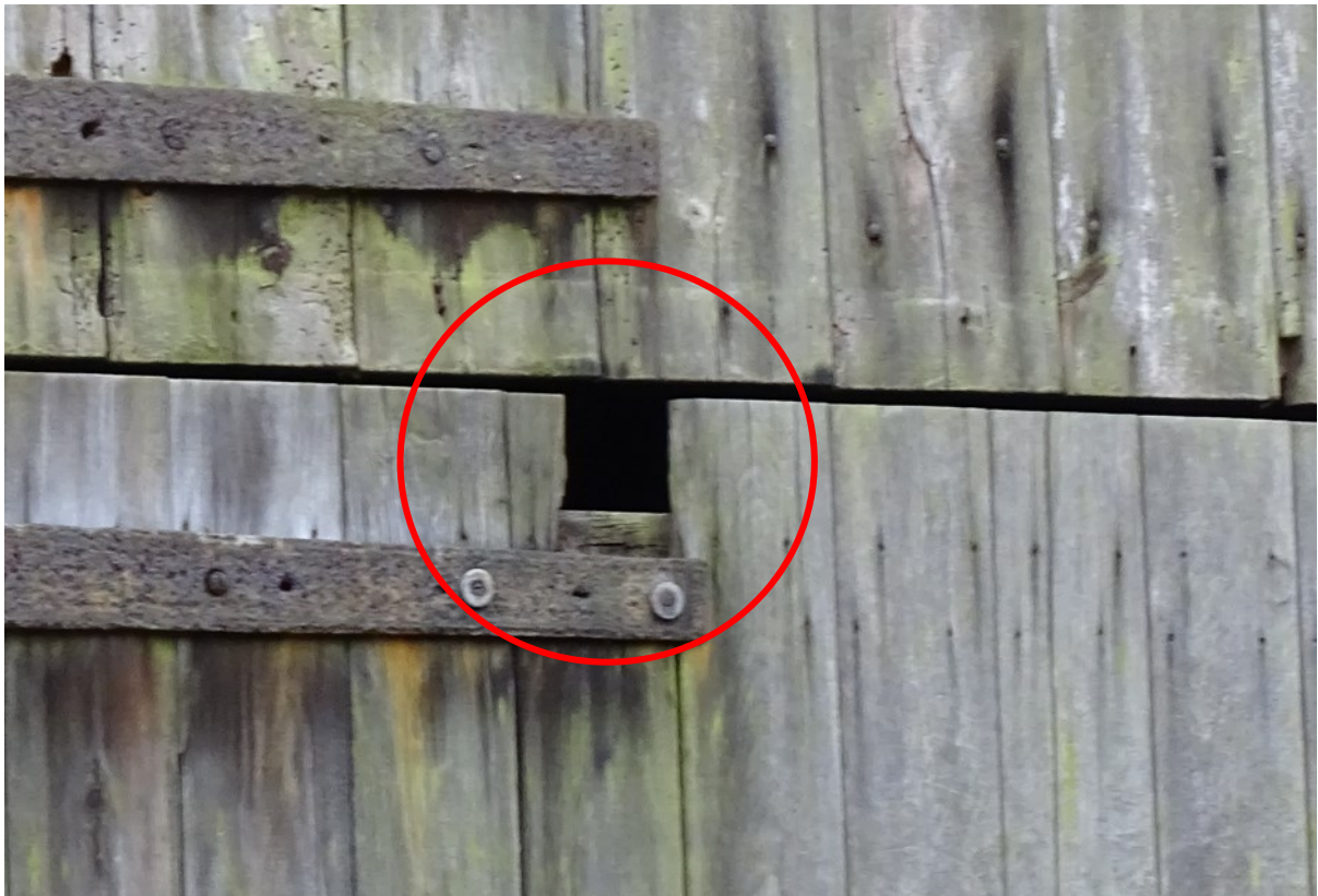
Image 14 – B1 – Example of gaps within the openings within the North areas of the structure which look to offer opportunities for both bats and nesting birds
