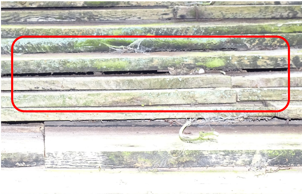
Image 15 – B1 – Gaps within the timber claddings to the North areas of the structure
