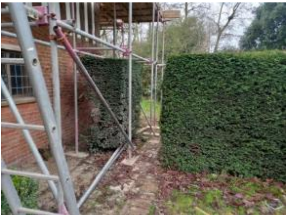
Plate 3.10: Gap in mature yew hedge (<1 m wide) through which building materials will be transported
