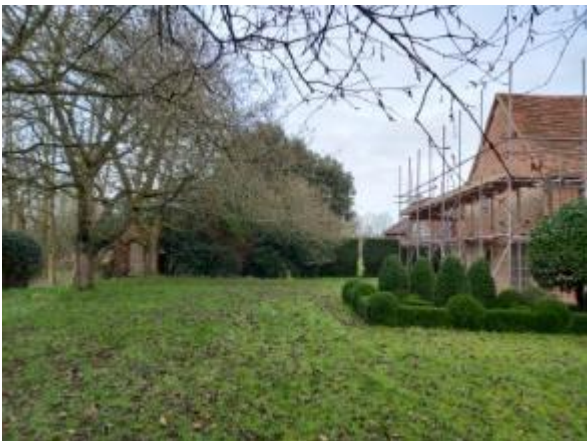
Plate 3.1: Western gable end of house, where the new extension will join, mown grass and cherry trees
