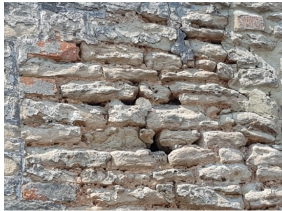
Photo 8: Gaps in stonework
