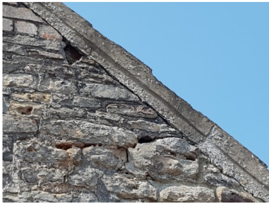
Photo 7: Gaps in stonework
