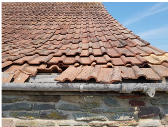
Photo 9: Damaged roof tiles
