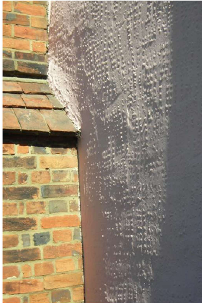
Fig. 11 Painted render with dotted patterning on a timber framed cottage, no. 16 High Street.
