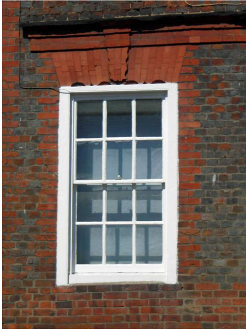
Fig. 12 Red and blue brickwork and rubbed brick decorative window head on no. 98 High Street
