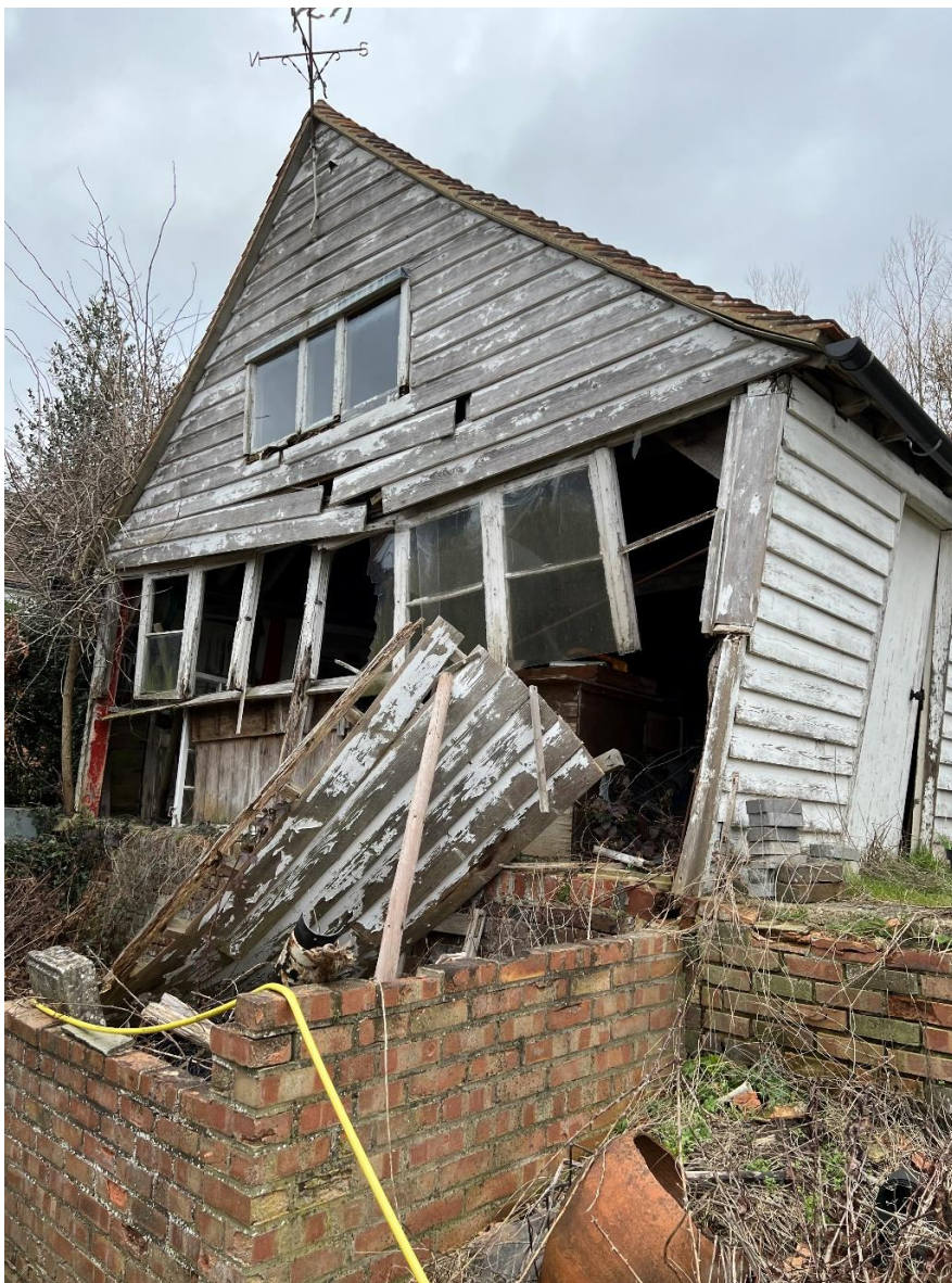
Fig 1: South elevation of dilapidated barn at Old Tong Farm
