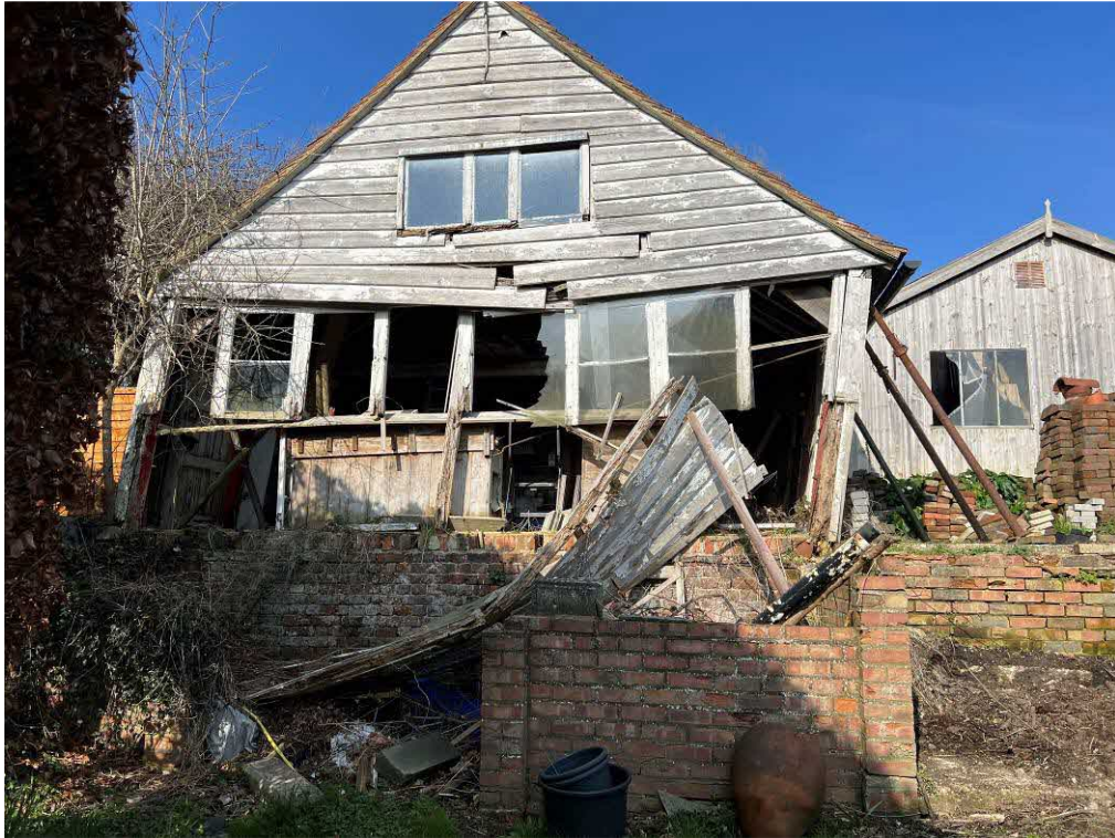
Plate 3 – South Elevation Showing Degree of Racking
