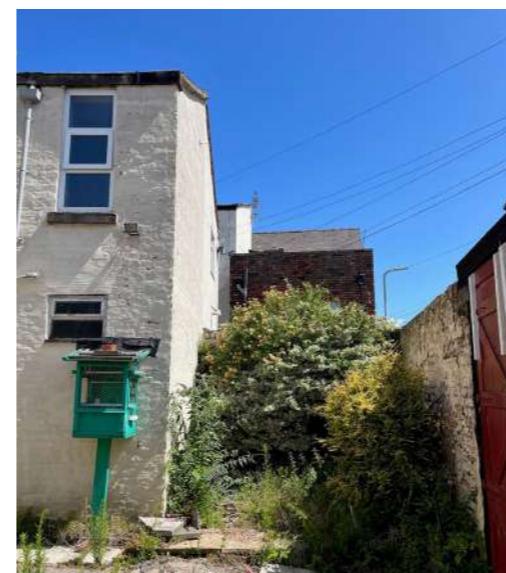
View towards the right side gable where open space can not be used due to over grown shrubs and an accumulation of waste material
