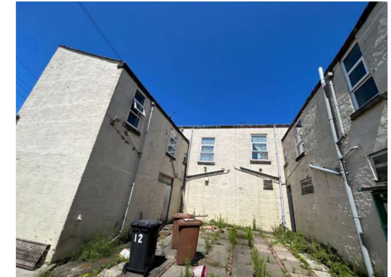
View from Dean Street showing the deteriorating elevations, crumbling render, unattractive window design and overgrowing landscape
