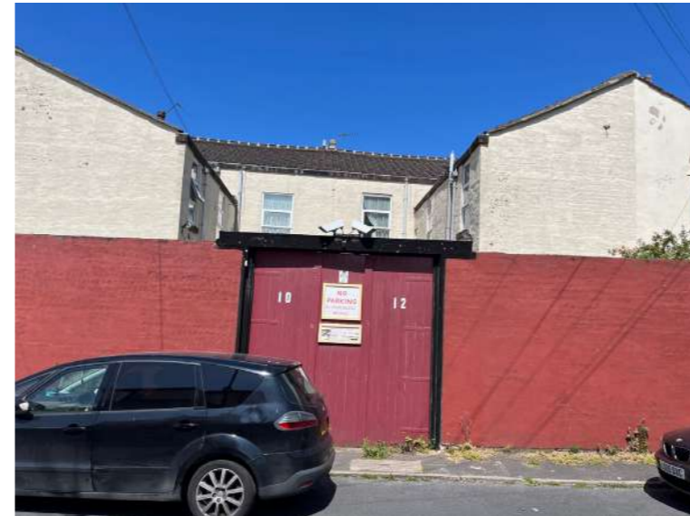
View from Dean Street where a large expanse of brickwork provides an unattractive and intimidating frontage to the street scene
