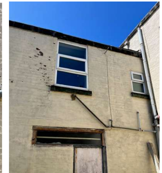
View to the left side gable with unattractive exposed drainage pipework, deteriorating elevation and window designs
