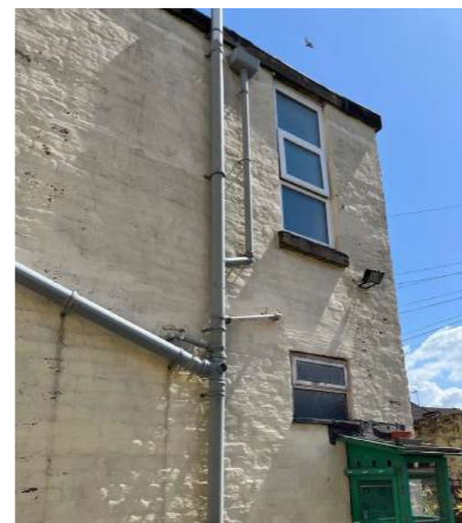
View to the right side gable with unattractive exposed drainage pipework and deteriorating elevation
