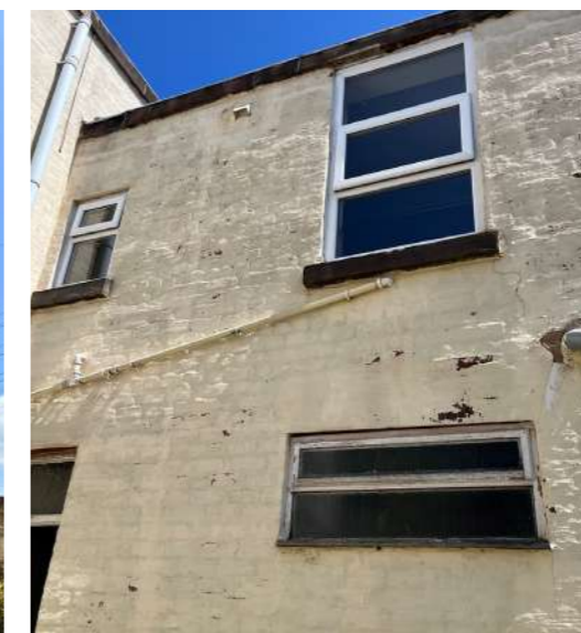
View to the right side gable with unattractive exposed drainage pipework and window designs
