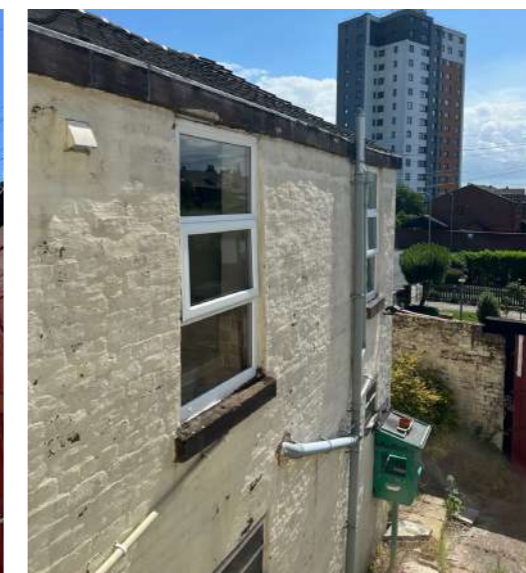
View towards the right side gable where a tall brickwork wal disconnects the site from the street and adjacent properties, creating an unwelcoming and intimidating frontage to the site
