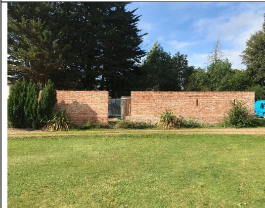
Fig 7. Barn as exists currently , eastern elevation. Note original opening and recreated vertical “arrow loop” type openings presumably originally for ventilation
