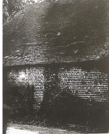
Fig 4. Evidence of kent clay tiles and random brickwork pattern based on a flemish bond
