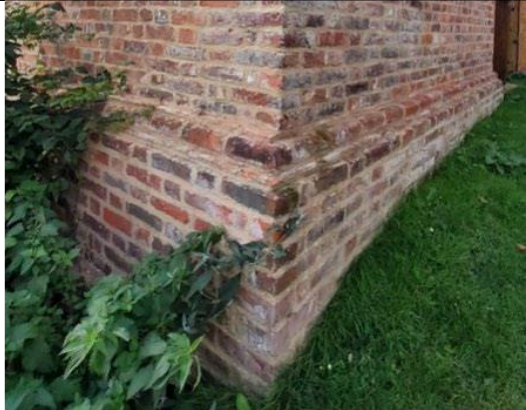
Fig 10. From the brick corbel course down is original brickwork and gives valuable clues to reconstruction elsewhere.
