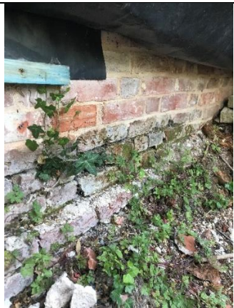
Fig 8. Brick detailing on southern gable end of north part of barn. Note both 18 th Century brickwork and new brickwork using reclaimed bricks and lime based mortar.
