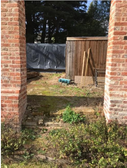
Fig 11. This opening is known to have existed as it was infilled with a modern yellow brick.
