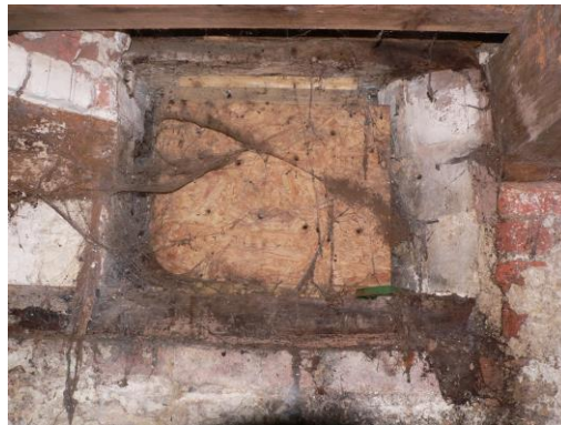
Copious amount of cobwebs found on cellar wall.
