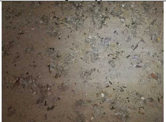
Photo 12 Natterer's dropping below joint in the tie beam/brace
