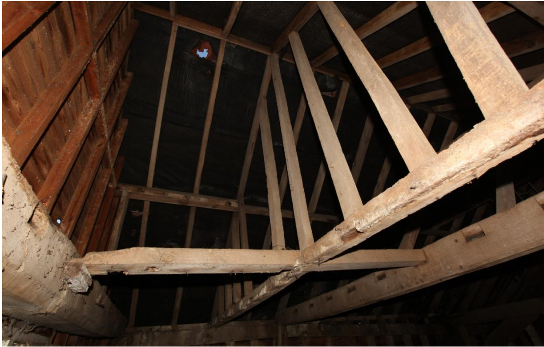
Illus. 19. The single ostensibly original first-floor ceiling joist that survives in the westernmost bay (A), tenoned between the tie-beam of the missing partition against the threshing barn on the right and the neatly chamfered and stopped binding joist that now forms the tie-beam of the gable on the left (seen from the south). This was incorporated into a later partition possibly of the 18 th century that may have enclosed a narrow stair opposite the southern entrance door to this bay.
