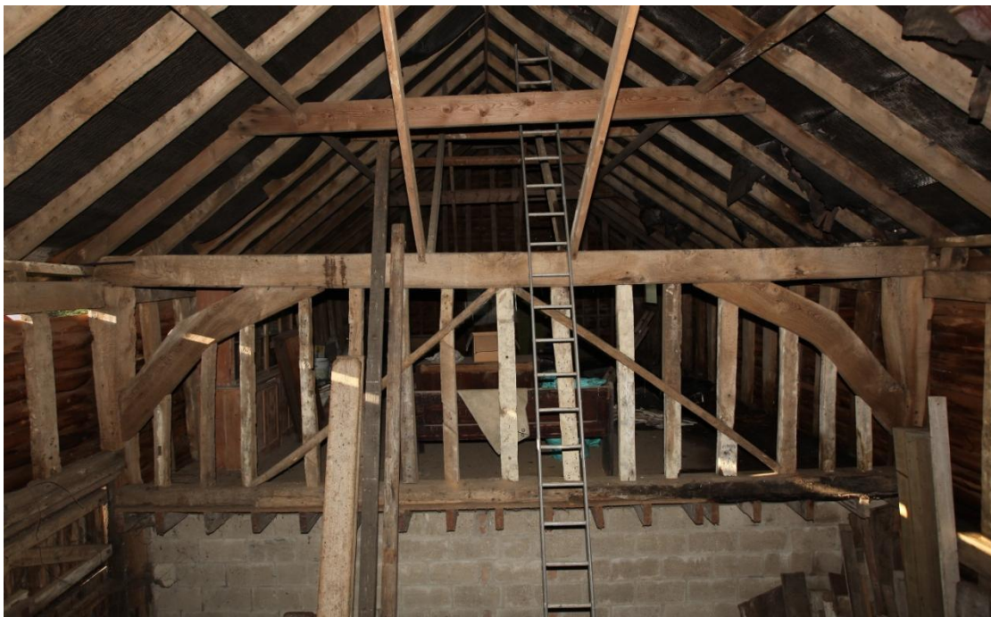
Illus. 12. The open truss to the west of the threshing bay (C) showing its impressive arch-braces with the 20 th century loft in bays A and B beyond (supported on block-work). The structure is a very impressive 23.25 ft in total width and its tie-beams lack mortices for queen or crown posts – indicating the original roof contained side-purlins.
