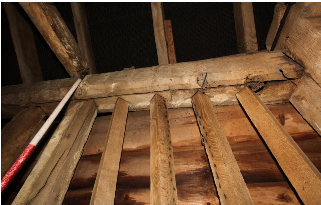
Illus. 24. The roof-plate above the southern window in illustration 23 contains a very narrow quarter-inch groove for a sliding internal shutter. Narrow grooves of this kind are usually seen only in high-status domestic houses which possessed finely made shutters of thin imported wainscot instead of the thick planks used in most cases.
