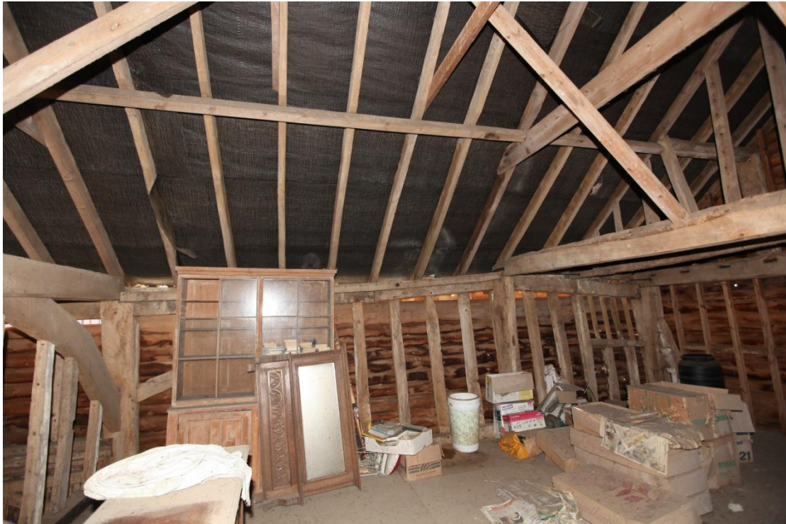
Illus. 21. The southern internal wall of bays B and A on the loft showing their intact framing with a window to the right and an original internally trenched brace to the left. Bay B was originally part of the threshing barn while the narrow bay A contained ground and first-floor rooms with ceilings that both extended beyond the present gable.
