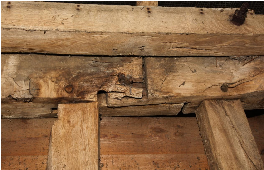
Illus. 22. A detail of the short face-halved and bladed scarf joint of late-16th and 17th century form in the southern roof-plate of bay B (to the right of the cabinet in illustration 21). Joints of this type first appeared in the final years of the 16 th century and replaced the earlier edge-halved and bridled form. It would be interesting to know which form was used in the farmhouse to establish whether the two buildings are exact contemporaries. The bolted reinforcing plate above is a 19 th or 20 th century addition.
