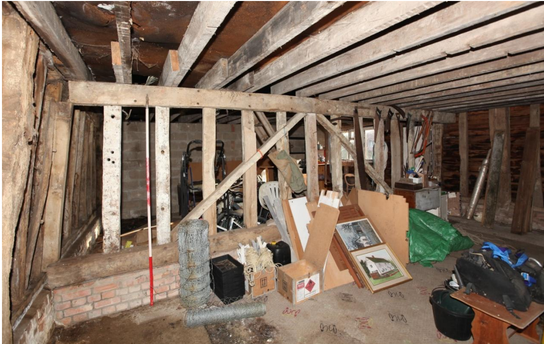
Illus. 13. The ground-floor partition beneath the 20 th century loft in bays A and B, as seen from bay A to the west. This consists entirely of re-used timber interrupted by diagonal primary braces and dates from the late-19 th century but now rests on a 20 th century brick plinth. It incorporates the mid-rail of the original partition between bays A and B (i.e. the floored stable and the threshing barn) which was initially tenoned to the storey posts approximately 0.5 m to the west of its present position.
