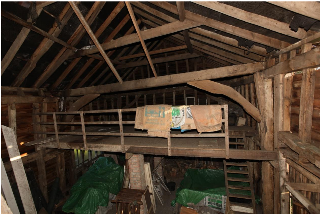
Illus. 8. The intact arch-braces and tie-beam of the open truss to the east of the threshing bay (C) showing the 20 th century loft in bay D beyond. The present clasped-purlin roof structure consists of re-used rafters with pine purlins and nailed collars in the typical manner of the late-19 th and early-20 th centuries.
