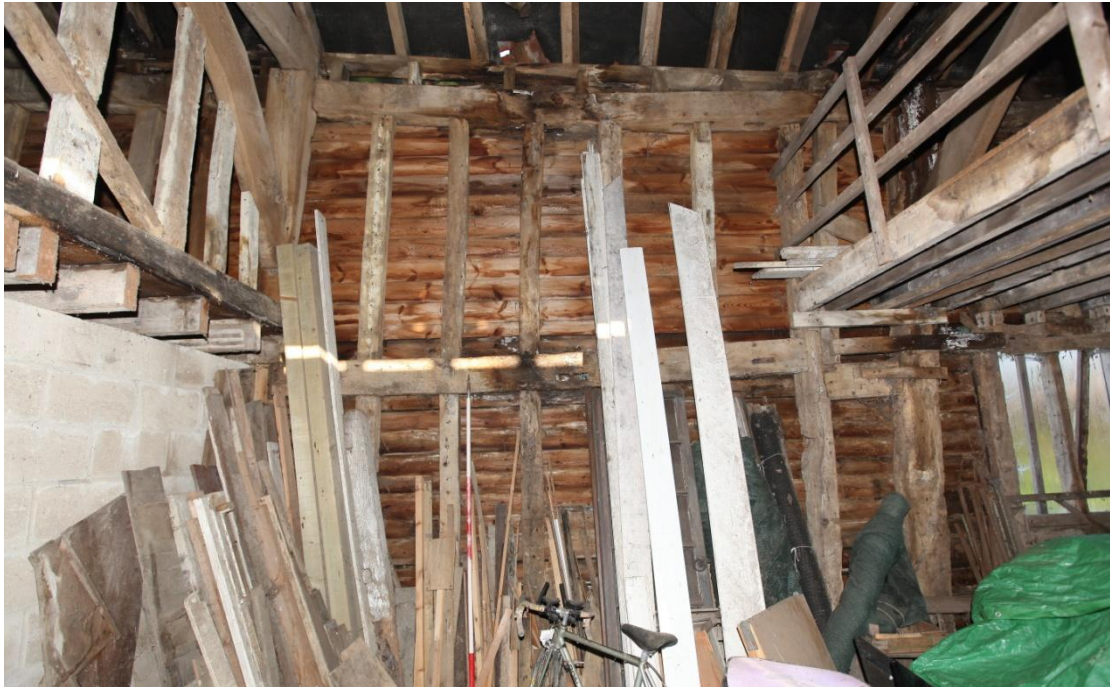
Illus. 7. The northern internal wall of the threshing bay (C). In contrast to the southern elevation the roof-plate here contains pegged mortices for original studs that formed a solid wall with a small central door beneath a mid-rail. A short section of original mid-rail survives to the right (under the loft) but the framing to its left consists of re-used timbers that were inserted to block a secondary doorway rising to the roof-plate. An original stud and a section of wall brace are visible above the original mid-rail.
