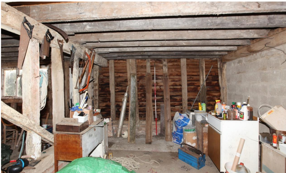
Illus. 14. The southern internal wall of the narrow westernmost bay (A) showing its storey post approximately 0.5 m to the right of the present partition on the left. The chamfered binding joist above the cement block-work of the gable to the right contains mortices for missing ceiling joists matching those in illustration 3, and the southern mid-rail contains evidence for an original door and window (illus. 15). Although this bay contained a ceiling initially the present tall-sectioned joists date from the 20 th century.
