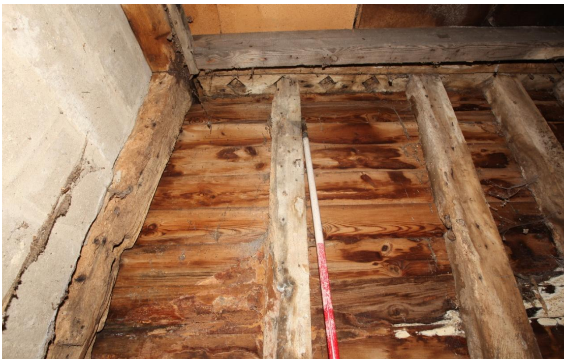
Illus. 16. The underside of the northern mid-rail of bay A showing evidence of another original window with four diamond mullions immediately opposite that in illustration 15. The corner post on the left and the stud on the right contain pegged mortices for the sill and a narrow groove for a sliding shutter is visible in the underside of the mid-rail.
