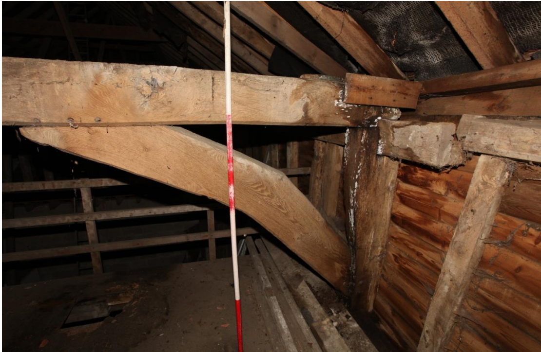
Illus. 11. The north-eastern corner post of the threshing bay (C) showing its heavy original arch-brace and the crude joint linking its roof-plate to that of the separate, later structure of the eastern bay (D). This consists of a simple tenon with a housed soffit but lacking a peg that projects from bay D in bay C. An identical joint lies in the southern plate. A large unpegged mortice 13 inches in height lies just above mid-rail level in the eastern face of the storey post. A similar but smaller mortice is visible in the southern post but at a slightly higher level. Both must relate to the predecessor of bay D.
