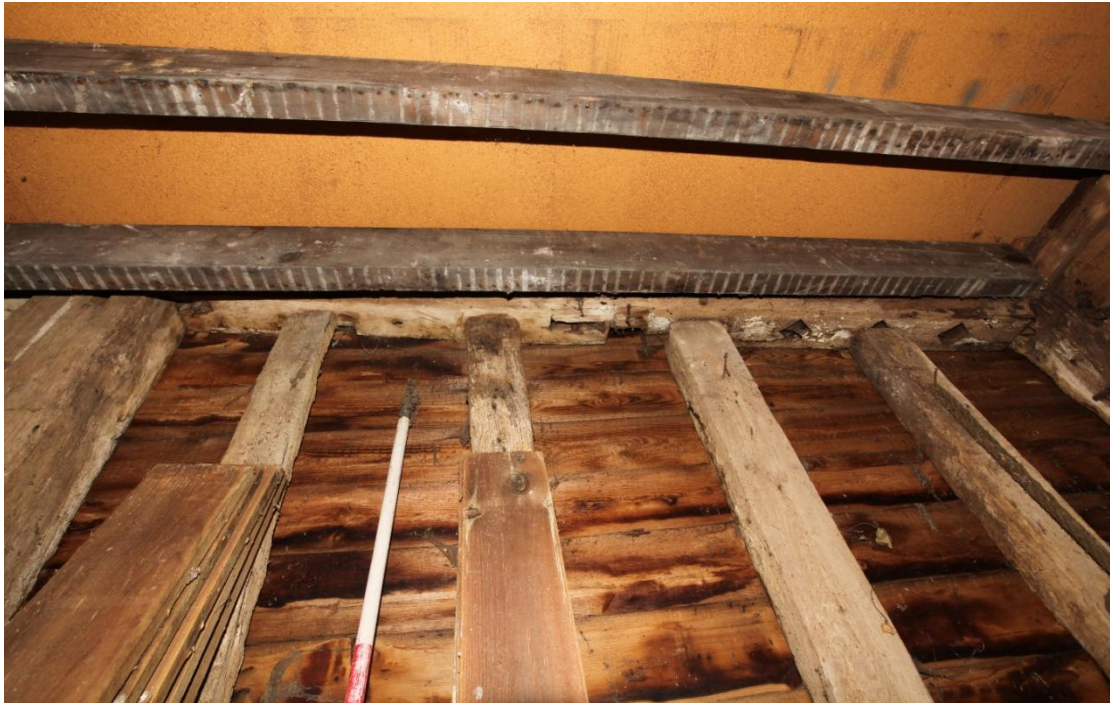
Illus. 15. The underside of the original southern mid-rail of bay A (illus. 14) showing three empty diamond mullion mortices for an original window to the right and a gap for an original entrance door against the storey post to the left. None of the four studs occupy their original positions, but the present corner post on the right contains a pegged mortice for the window sill. A small pegged mortice abutting the post held the missing door jamb. Of the four windows the bay this is the only one with three rather than four mullions and without a shutter groove – as the door restricted space.
