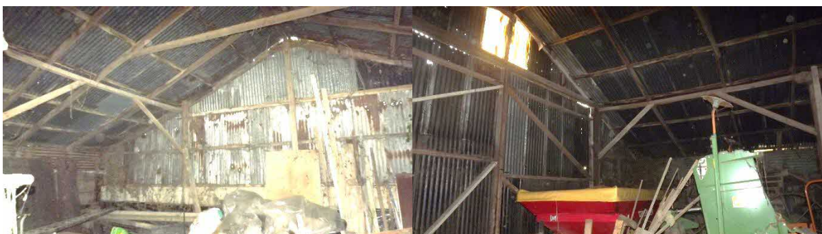
Fig 5 & 6. Internal view of west gable (left) and east gable and timber frame (right)
