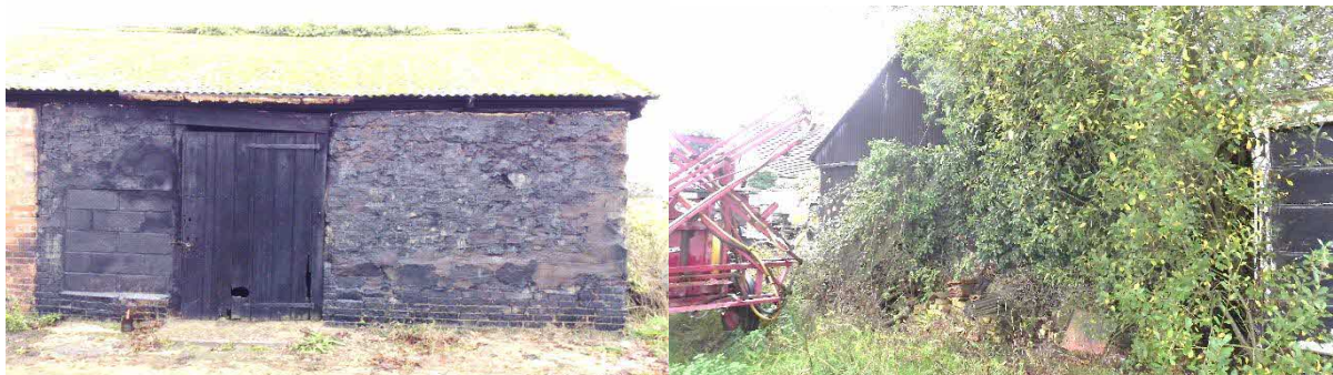
Fig 9 & 10. East elevation with tar coated clay lump (left) and overgrown north gable end (right)
