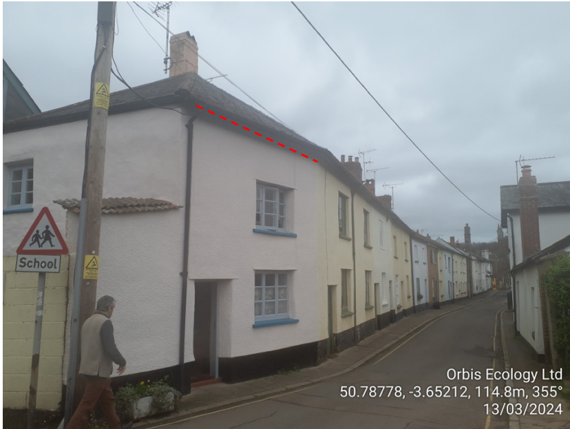
Area with nesting material observed from within the roof void
