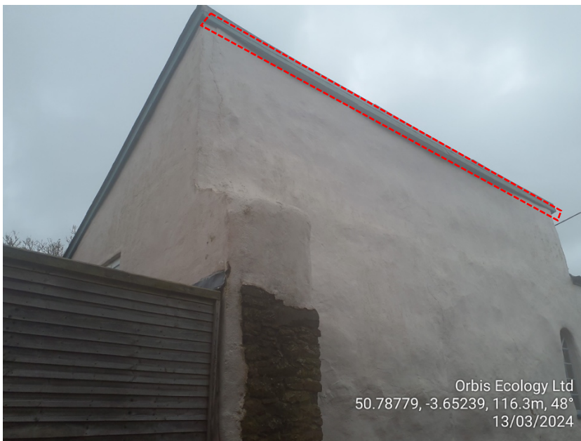
Gaps under fascia board on single pitch rear roof
