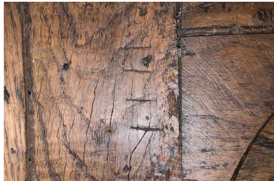
Carpenters marks on wood panelling (top) and above the South fireplace (bottom)
